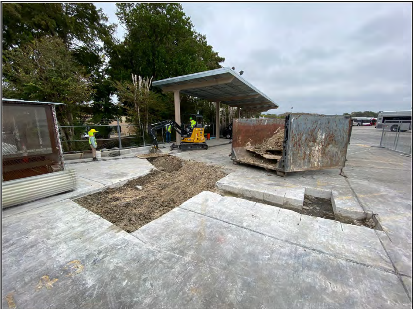
Figure 4-2. Electrical conduit trench locations. Note partially completed bus charging area and San Pedro Creek in background, thick pavement overlaying project area.
