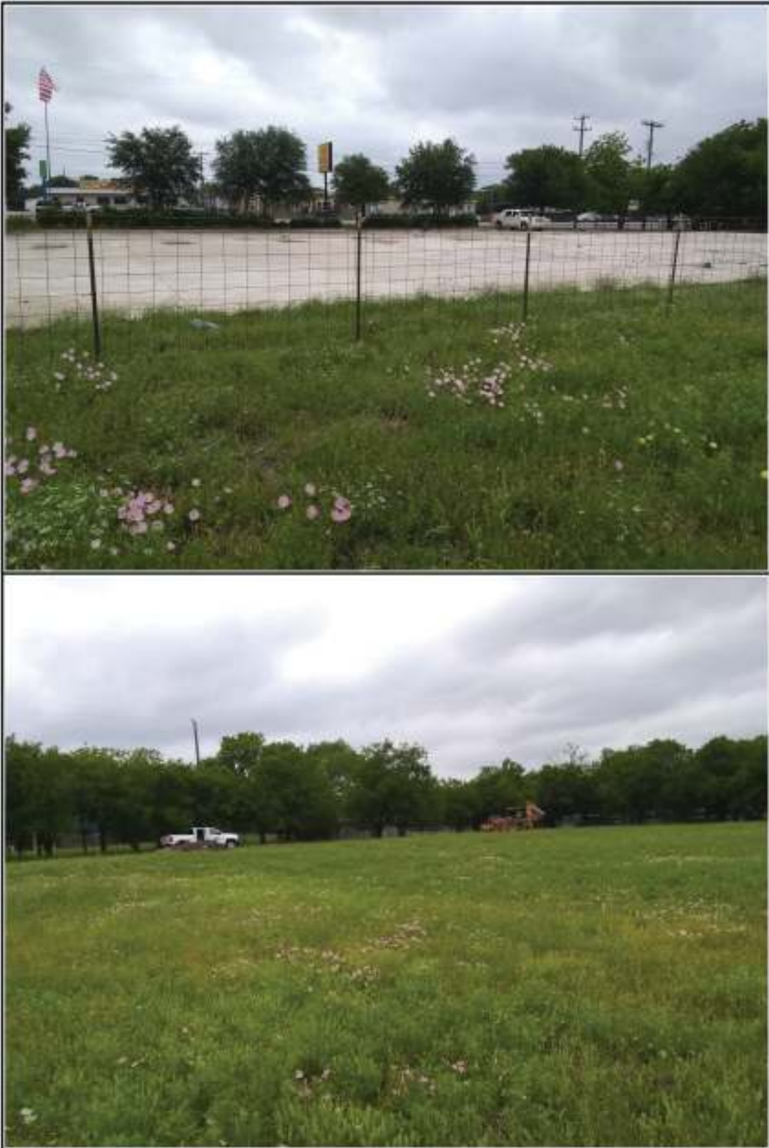
Figure 1-3. The southeast paved portion of the project area (top). The open field portion of the project area was trenched with a backhoe (bottom).
