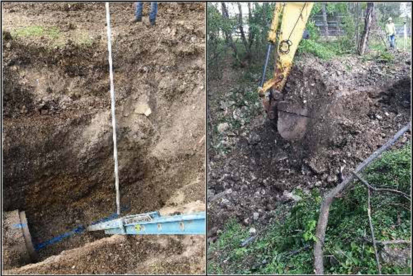
Figure 4-7. Images showing construction fill used to build up and stabilize the landform in the northwest portion of the project area (storm drain) and the outlet to Beitel Creek.
