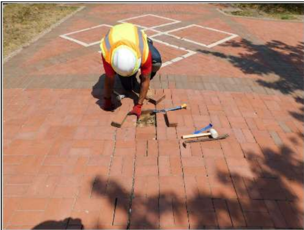
Figure 3-1. Removal of pavers on the west side of the Benjamin Milam monument.
