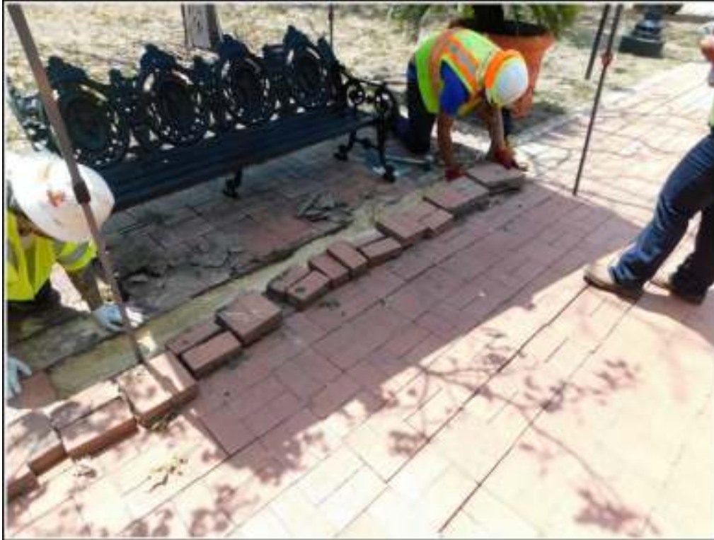
Figure 3-2. Paver repair on the west end of the park facing San Saba Street.
