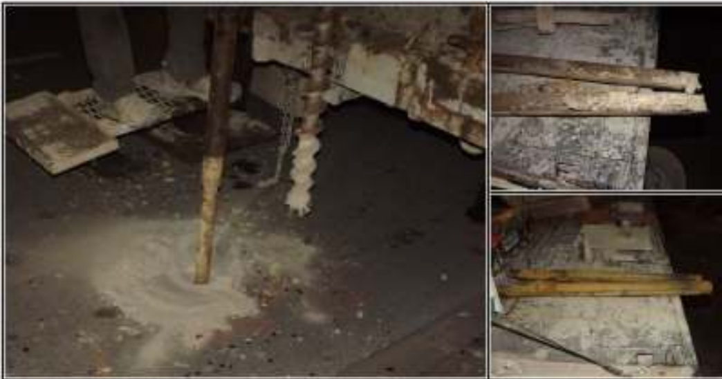
Figure 4-3. Boring of B-3 in progress; sample 1 (top right) and sample 7 (bottom right).
