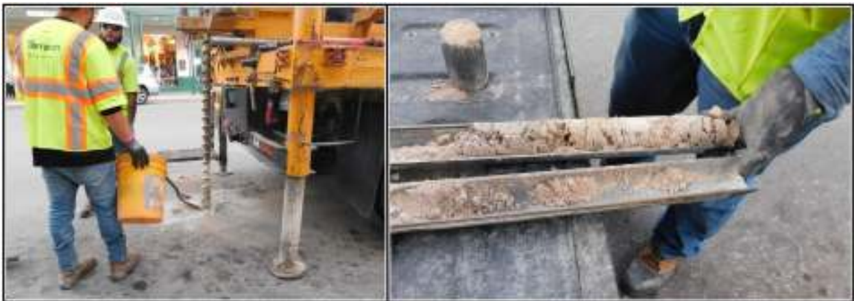
Figure 4-3. B-1: left) boring in progress, view southeast, and right) first core sample.
