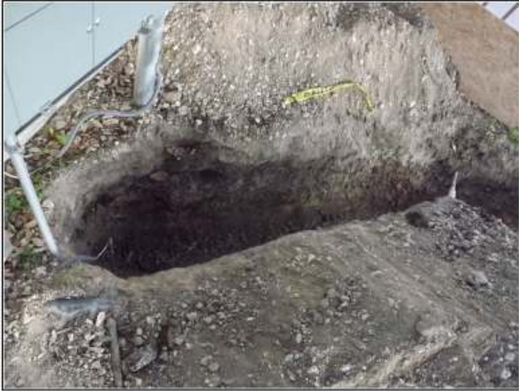
Figure 3-1. Trench Section 1 from transformer pad running west to east, connecting to Trench Section 2.
