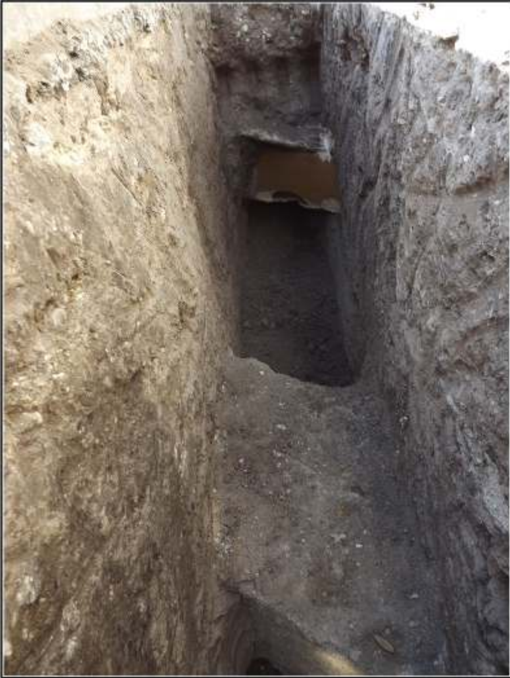
Figure 3-4. Northeastern portion of Trench Section 3 that connects to Trench Section 2 beneath sidewalk.
