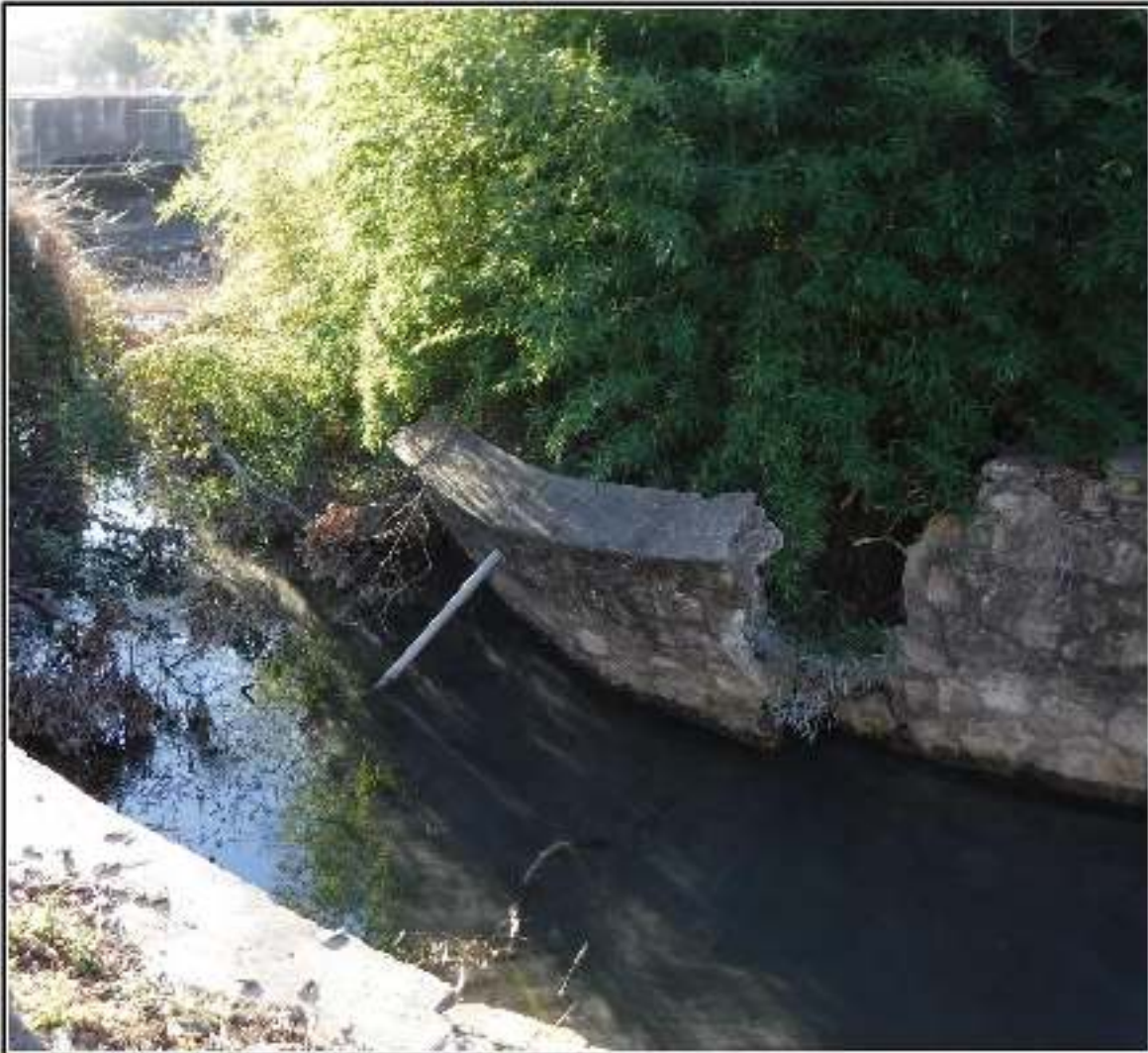
Figure 4-1. A photograph showing the collapsed canal prior to stabilization (looking southeast).
