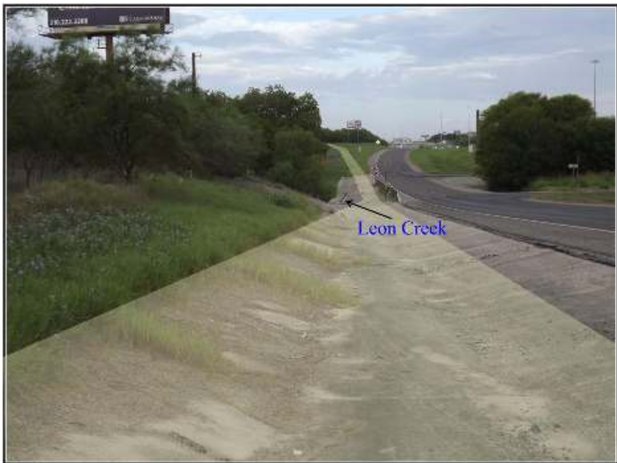
Figure 4-2. The APE (highlighted) near ST 4 leading to Leon Creek. View to the east.
