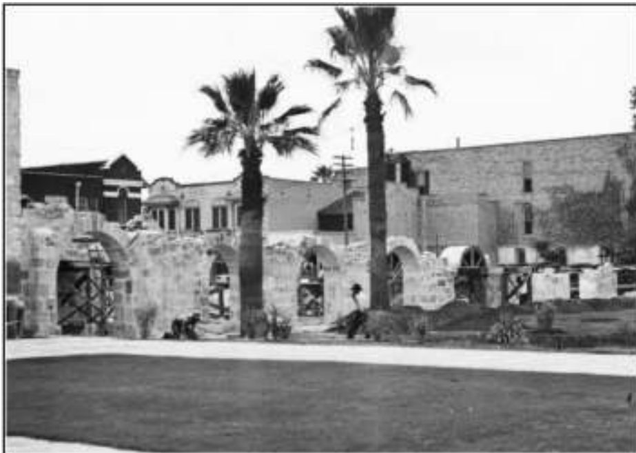
Figure 2-7. Photograph of arcade construction in September 1934. Original San Antonio Light caption: "Construction of the Alamo Arcade, with arches evocative of the conventos at Mission San Jose and Concepcion" (courtesy of UTSA-ITC, San Antonio Light Collection L-0342-E).
