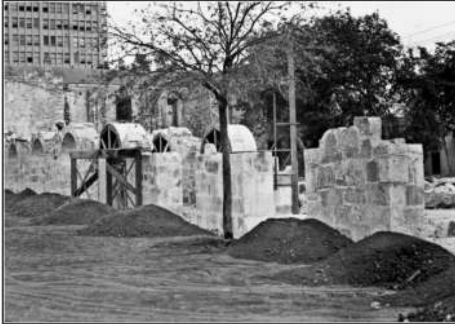
Figure 2-6. Photograph of arcade construction in September 1934. Original San Antonio Light caption: "Weathered limestone, salvaged from buildings previously located on the site, is used for the arcade" (courtesy of UTSA-ITC, San Antonio Light Collection L-0342-D).
