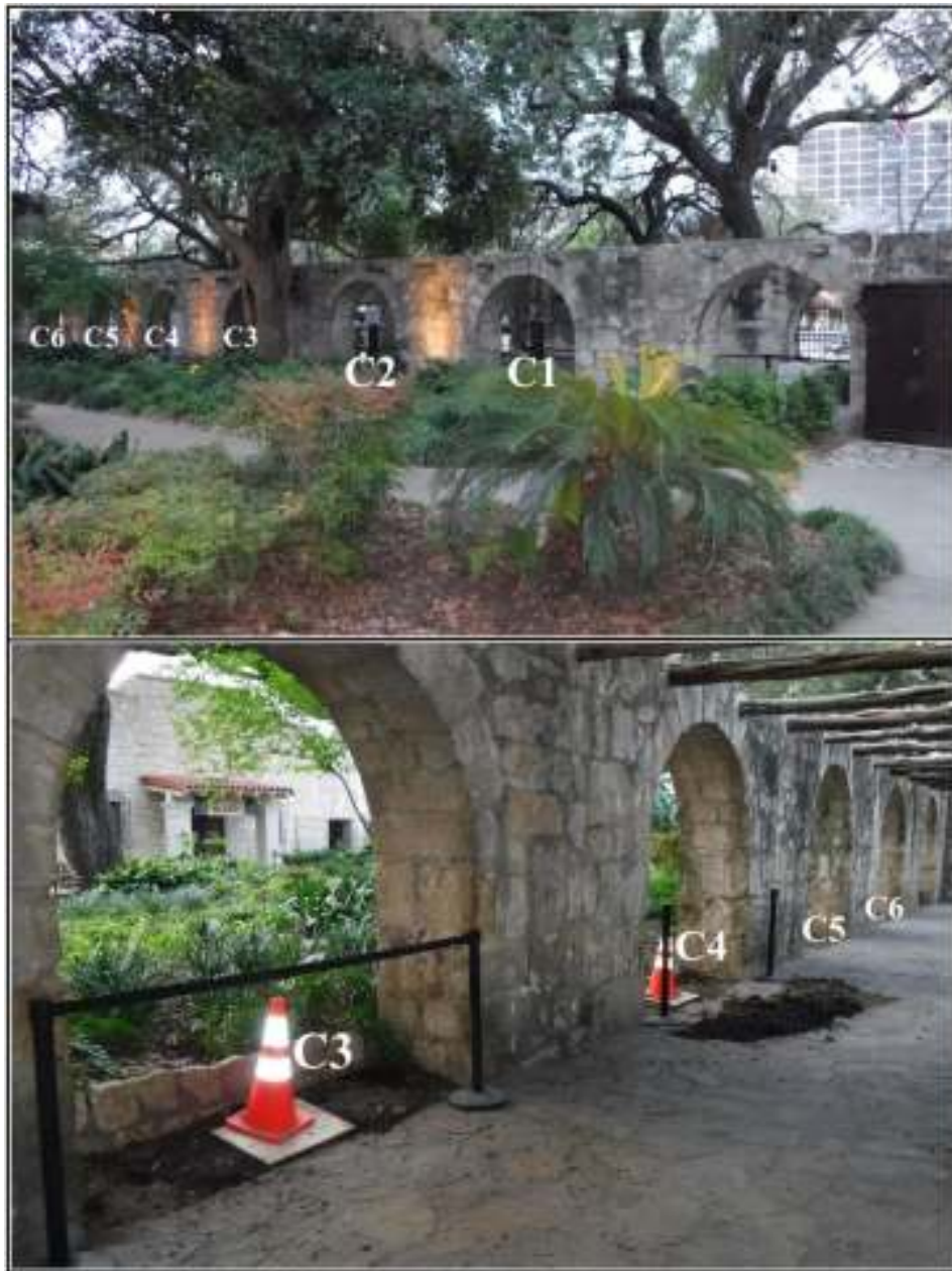
Figure 4-1. Project area showing a view of Alamo Arcade. Exterior (top) with first two (C1 and C2) cannon installed and locations for cannon C3 through C6. Interior (bottom) with holes for C3 and C4 completed and locations of C5 and C6 (view south).
