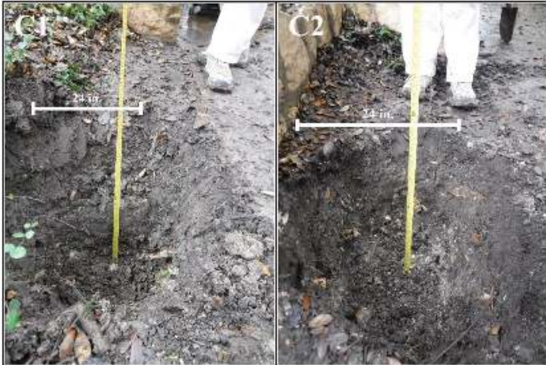
Figure 4-2. C1(left) and C2 (right) holes excavated to 24 in. (61 cm) below the surface.
