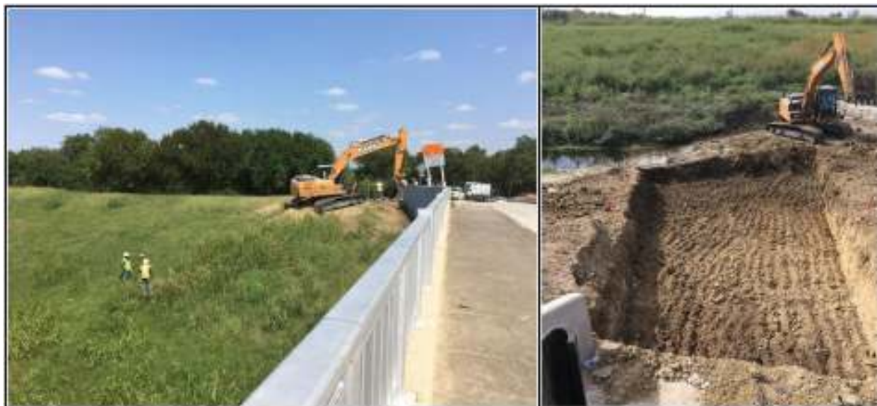
Figure 4-7. Beginning of the trench excavation for storm drain on Espada Road northwest of the Espada Acequia in Area 3 (left). The excavated storm drainage pipe outfall to Six-Mile Creek (right).
