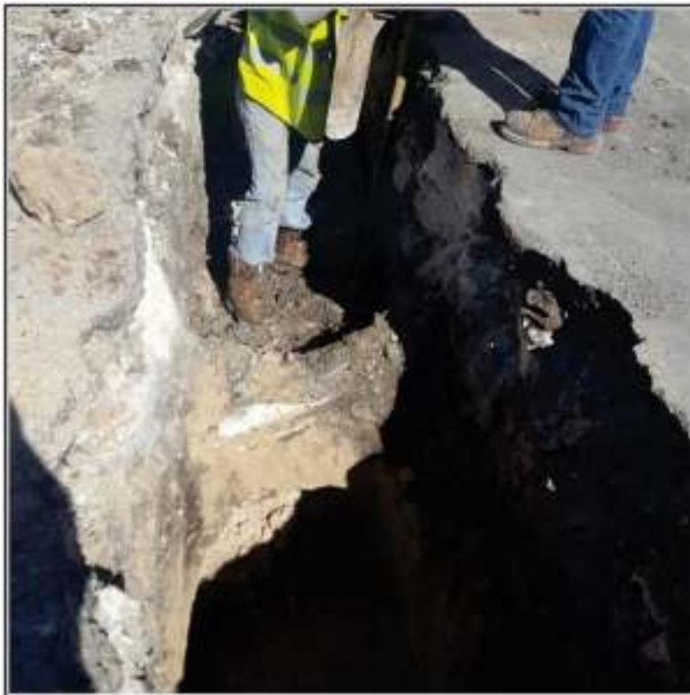
Figure 4-3. Trench 2 excavated to the west of Trench 1 and associated with SAWS utilities.
