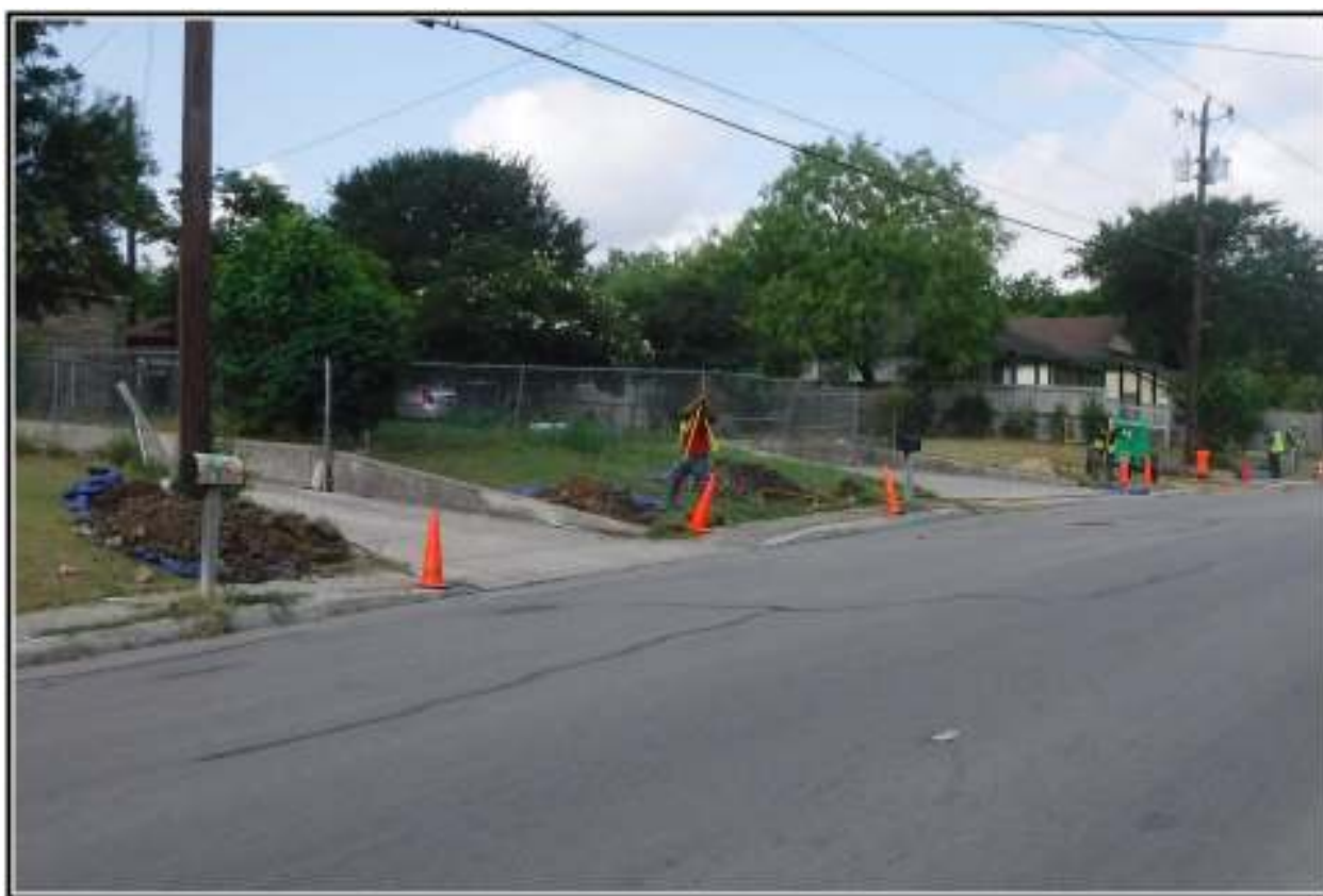
Figure 4-1. Hand-excavated trenches along the 500 block of Yucca Street, south side (view southwest).
