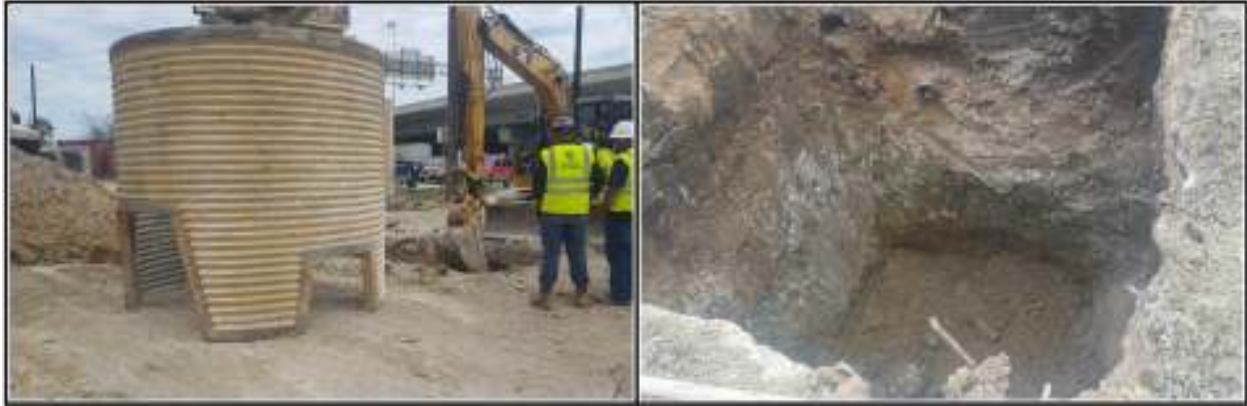
Figure 4-2. Excavation for manhole (left). Soil profile of excavation showing clay with caliche (right).
