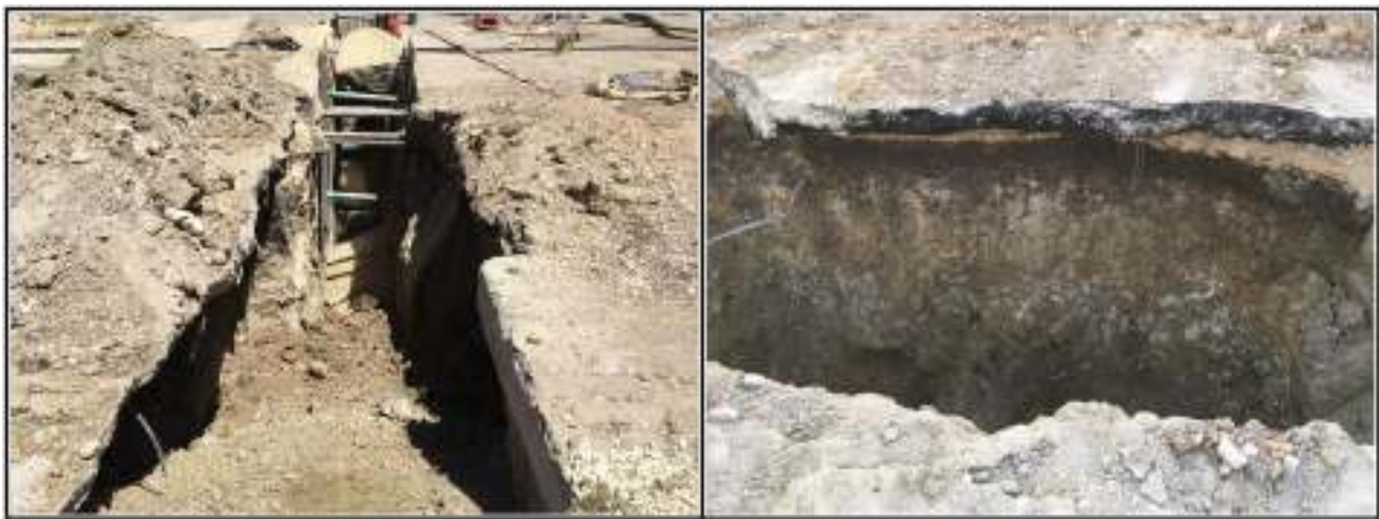
Figure 4-3. Excavation for sewer line showing evidence of previous construction (left). Image on the right shows a similar soil, clay with caliche, as observed during the manhole excavation.
