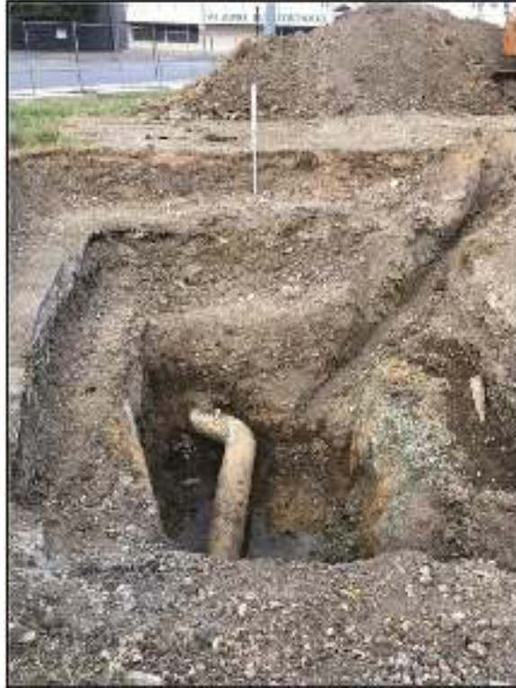
Figure 4-2. Large access pit excavated at south end of CNG line install, view to the southwest; existing CNG line exposed at approximately 3.66 m (12 ft.) below the surface.
