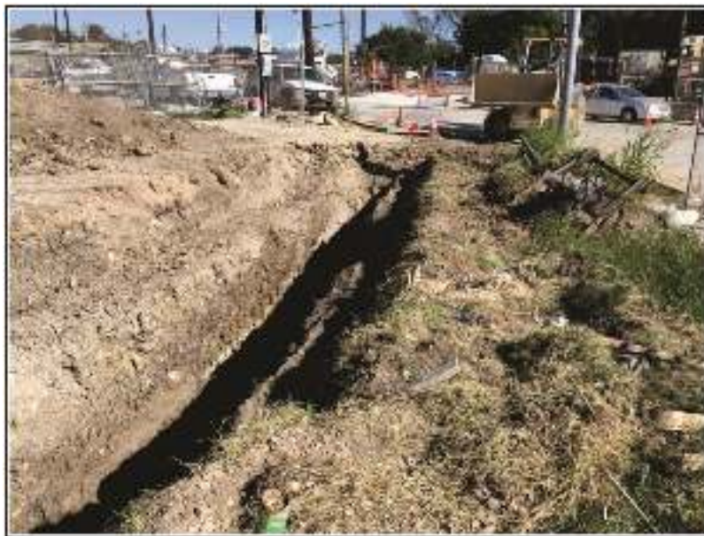
Figure 4-3. CNG trench at south end, view to the northeast; heavily disturbed strata.
