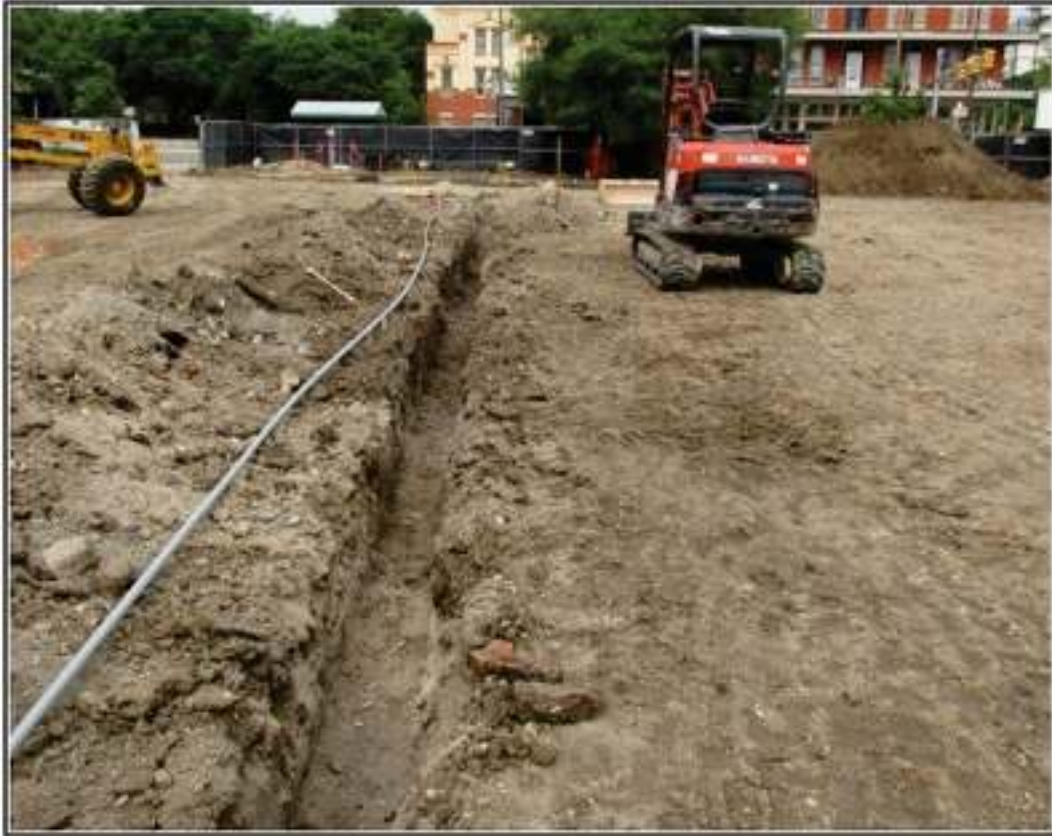
Figure 1-5. Trenching between pier holes. Note red and buff colored brick fragments on either side of the trench in foreground, April 12, 2016. View to the west.
