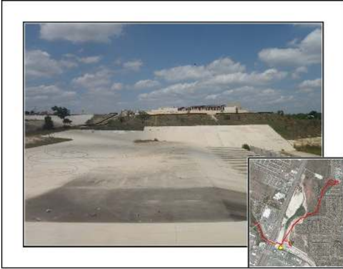
Figure 4-9. Dam and concrete apron at crossing of Culebra and Helotes Creeks. Inset shows approximate location on trail.
