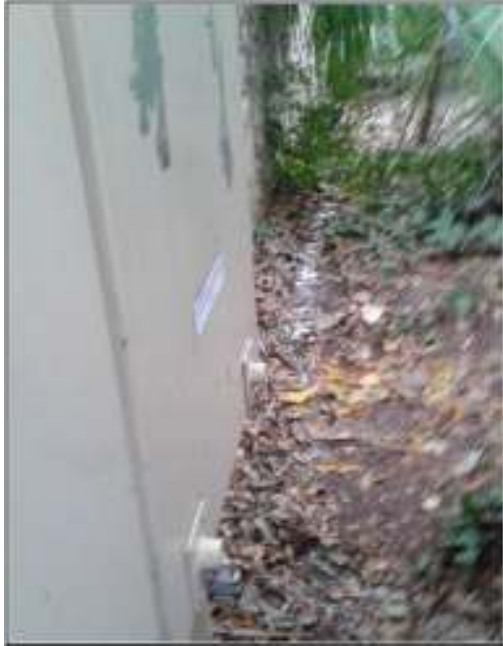
Figure 4-2. Existing circuit breaker box on north wall of complex and chalk-line indicating orientation of proposed trench.
