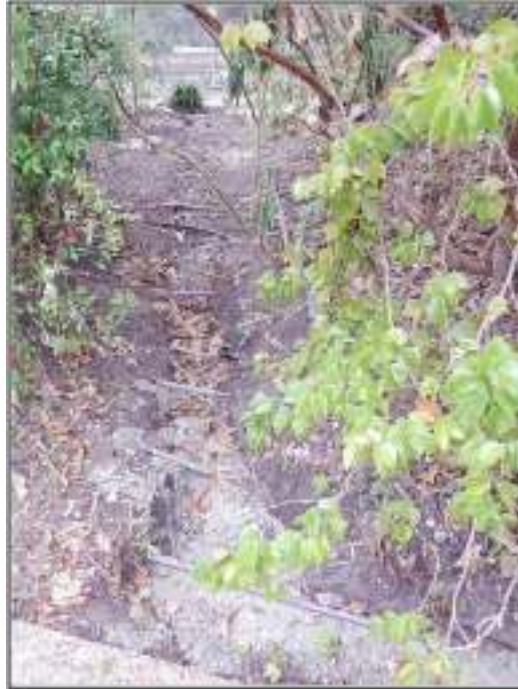
Figure 4-6. Conduit trench with pre-existing utility and irrigation lines, looking toward north wall of the complex.
