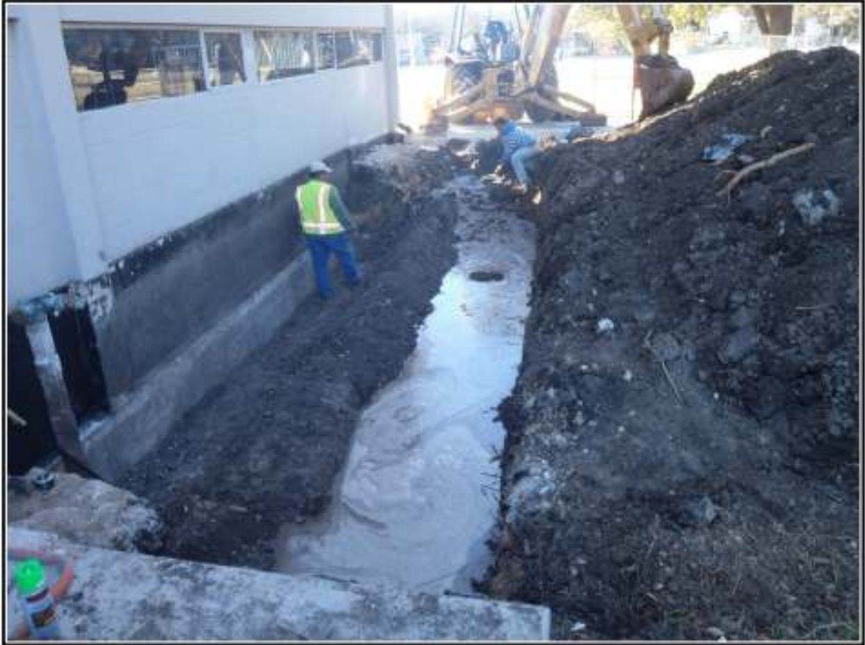
Figure 4-4. Trench 1 flooded along the 1.2-m deep side.
