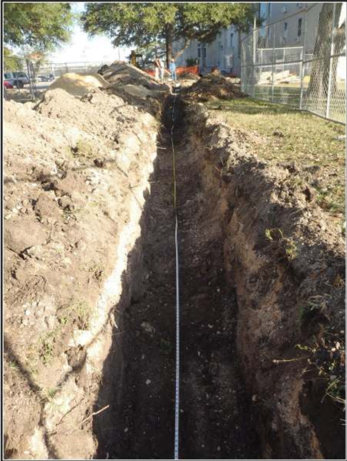
Figure 4-8. Trench 2 complete (facing east). View from grated drainage gutter towards the Playhouse.
