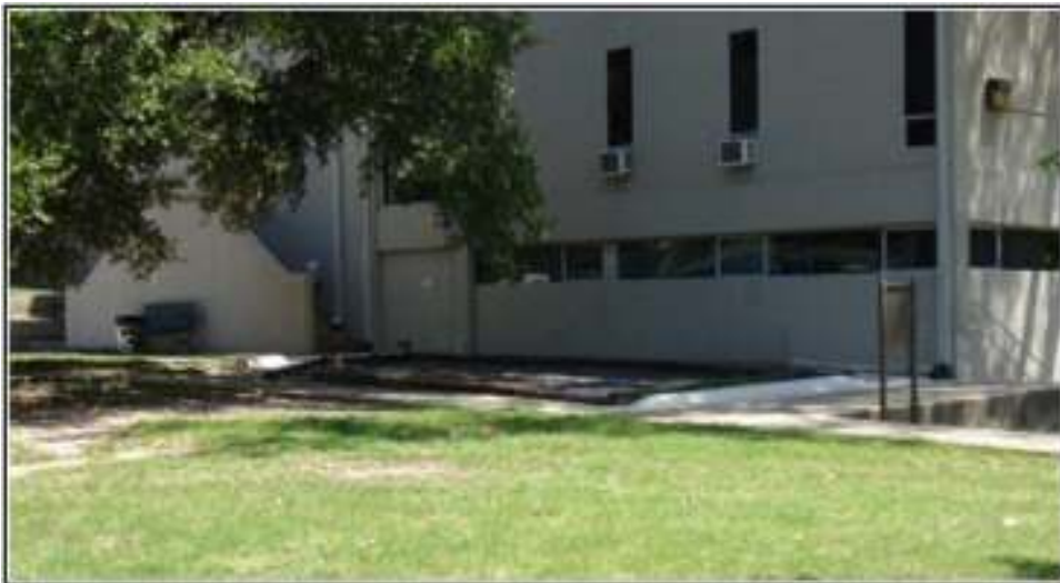
Figure 1-3. The northwest portion of the Playhouse showing the three downspouts to be redirected.
