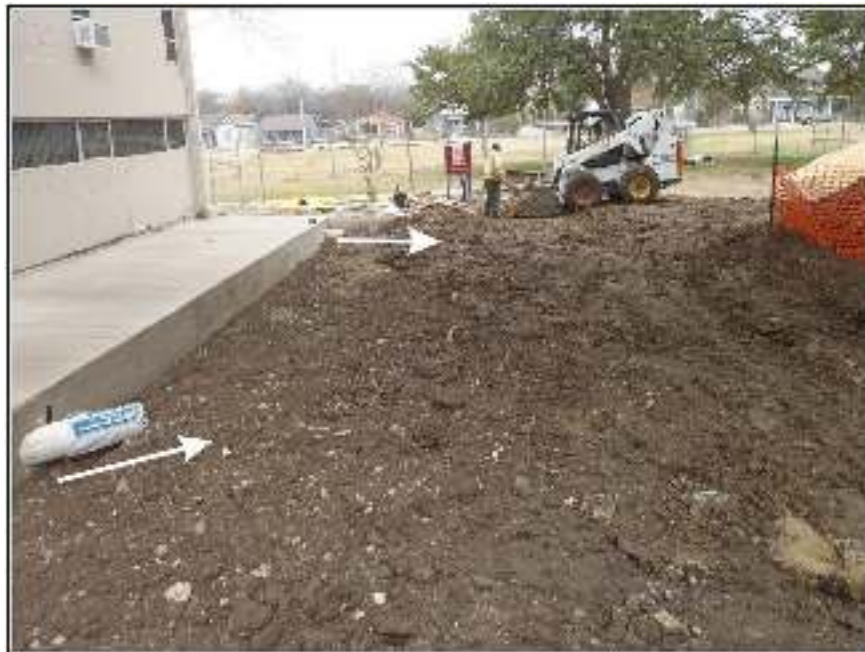
Figure 4-6. New sidewalk against north wall of Playhouse. Note drainage pipes extending from sidewalk.
