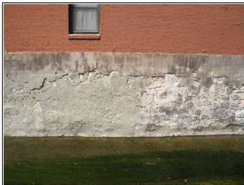
Figure 5-27. Original stone wall visible under peeling cement veneer, west bank of river just north of Dolorosa Street.
