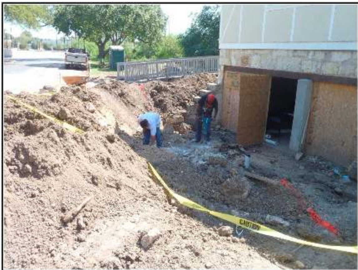
Figure 4-1. Excavated area to the north of the Borglum Studio building showing entrance to garage. Looking east-southeast.
