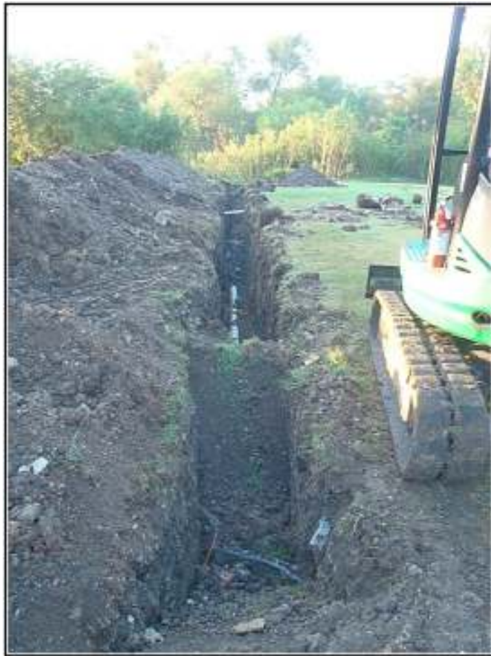
Figure 4-4. View of Trench 2 extending from near the structure to the Catalpa Pershing Channel in the background.
