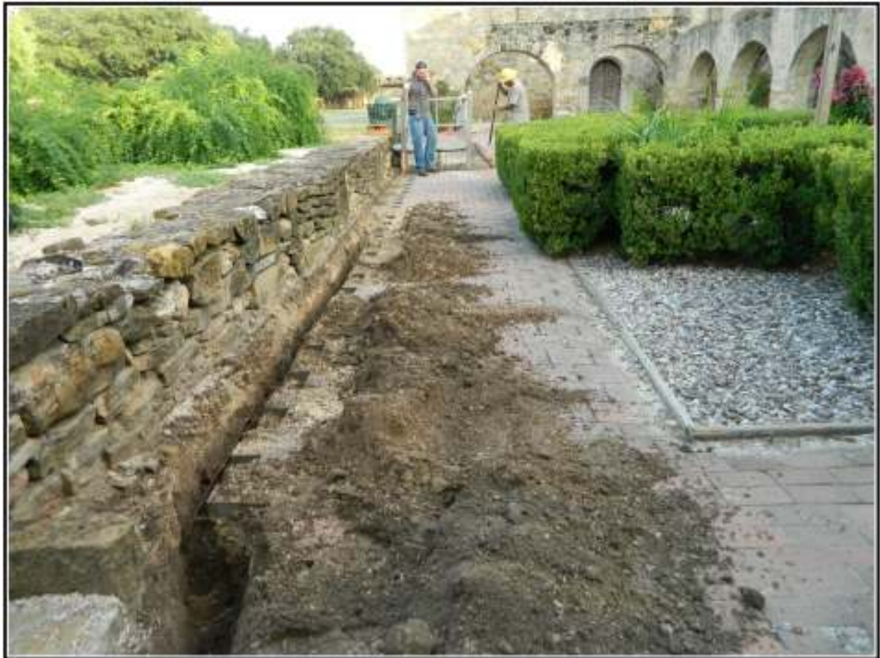
Figure 4-3. Excavation of Trench 5 along the inside of the retaining wall bordering the convento.
