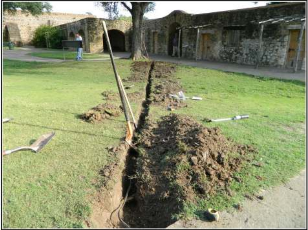
Figure 4-7. Trench 2 running from in front of the church to a junction box next to the tree.
