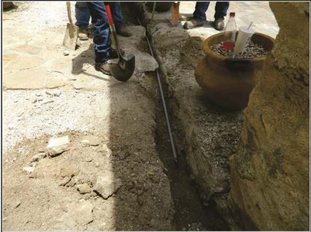
Figure 4-4. Trench 7 on the inside of stone foundation near back entrance to church.
