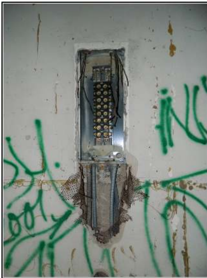
Figure 6-11. Fuse box noted on the main floor of the hospital.
