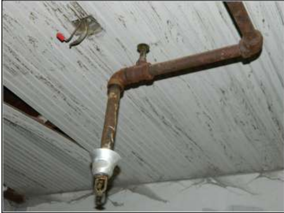
Figure 6-12. Example of the sprinkler system present throughout the hospital.
