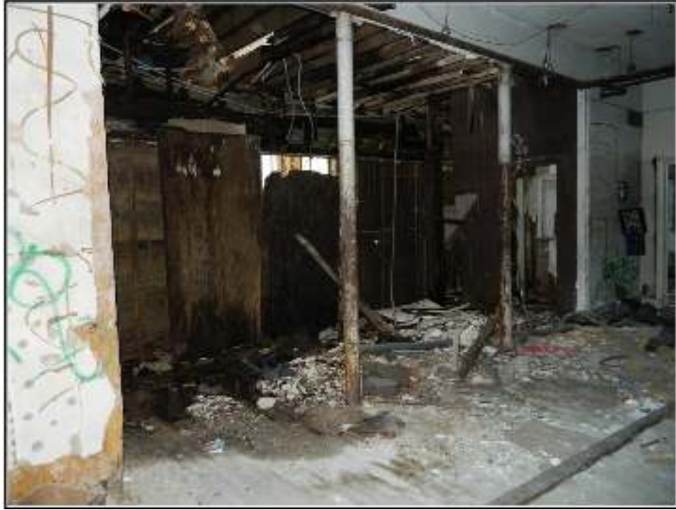
Figure 6-8. The interior of the Good Samaritan Hospital at the main entryway to the first floor.
