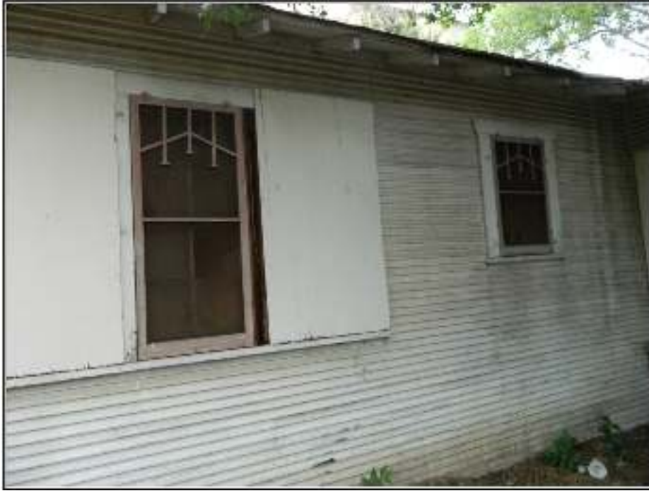
Figure 6-18. Decorative screens covering the windows of the eastern side of the house.
