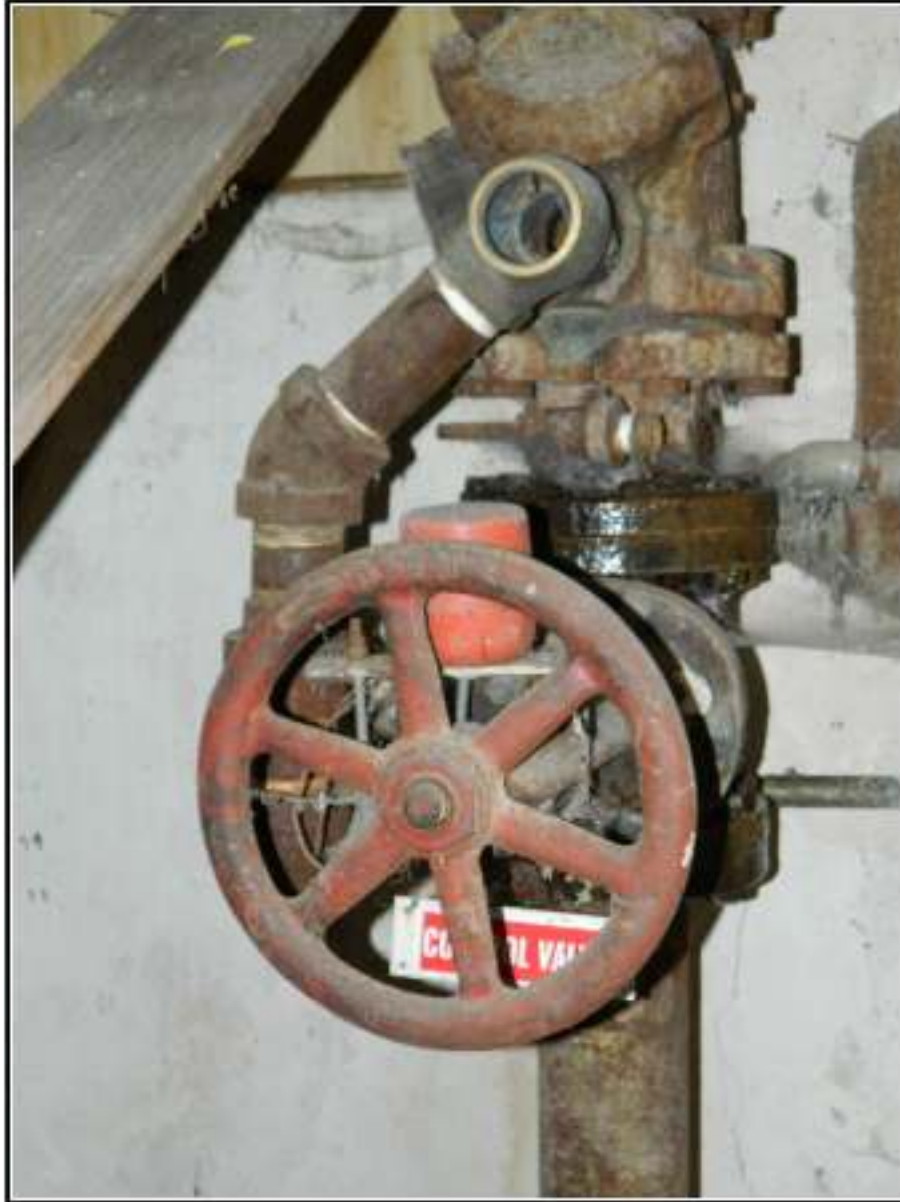
Figure 6-14. Water line and valve located in the northern room in the basement.
