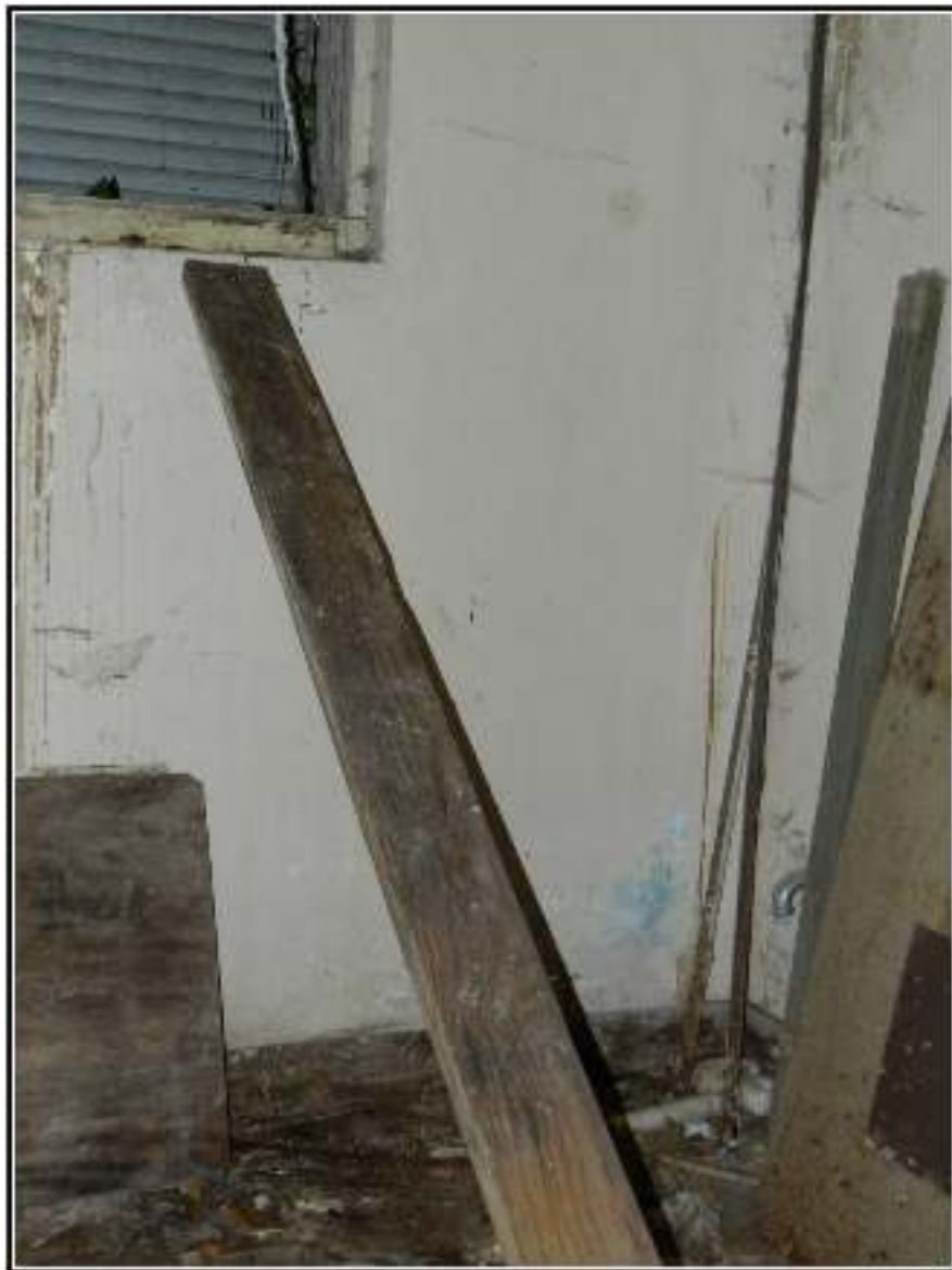
Figure 6-10. Room at the Good Samaritan Hospital in the basement that had an open window and plank.
