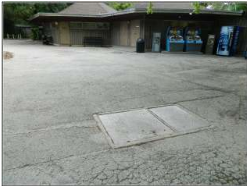
Figure 4-11. Subsurface electrical conduit box.
