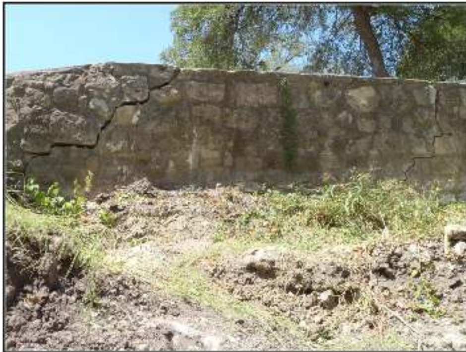
Figure 5-6. Portion of the currently standing Lily Pond wall near the fragments that were encountered in the backhoe trench. Note the cracks that indicate the unstable nature of the current wall.
