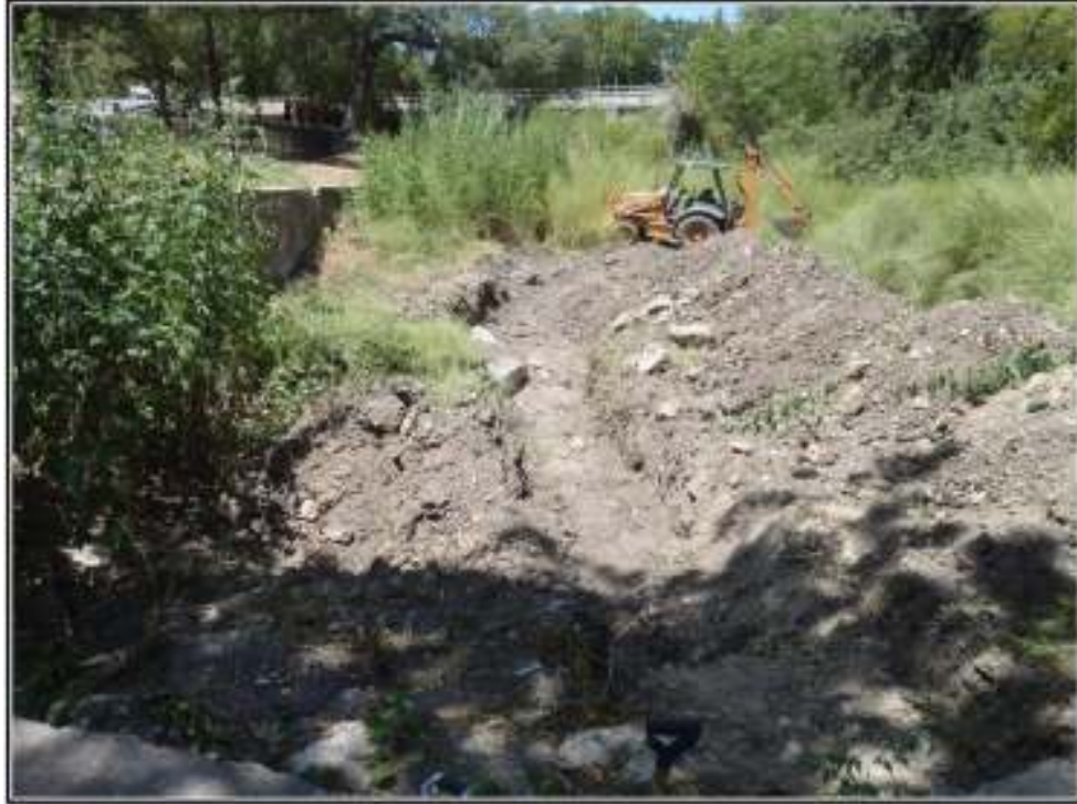
Figure 5-3. Entirety of the backhoe trench excavated within the Lily Pond. Rock wall fragments were encountered in the mid-portion of the trench.
