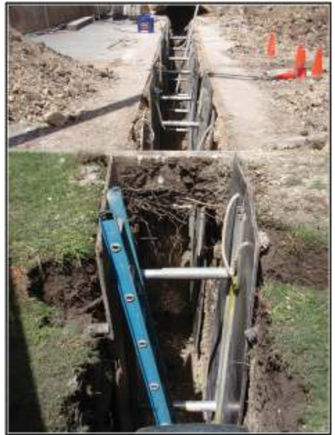
Figure 3-6. Storm Sewer Trench showing the expansion plates obstructing a clear view of the wall profile.
