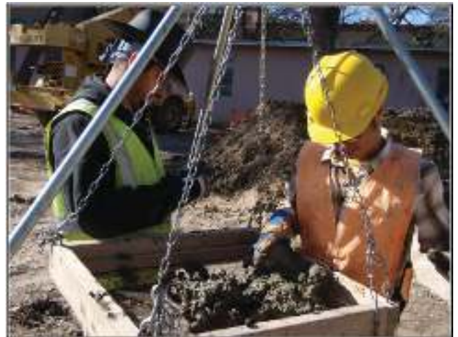
Figure 3-4. CAR staff screen excavated materials from pier borings in the footprint of the new extension.
