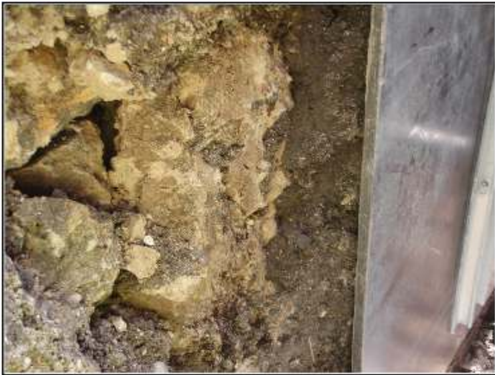
Figure 3-7. Feature 1 in north wall of Storm Sewer Trench in the vicinity of the second Alligator Garden.
