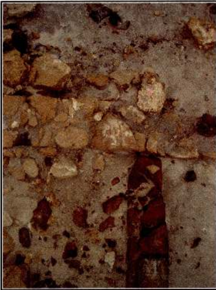
Figure 21. Intersection of the cross-wall between Rooms 2 and 3 and the south wall of the rooms.
