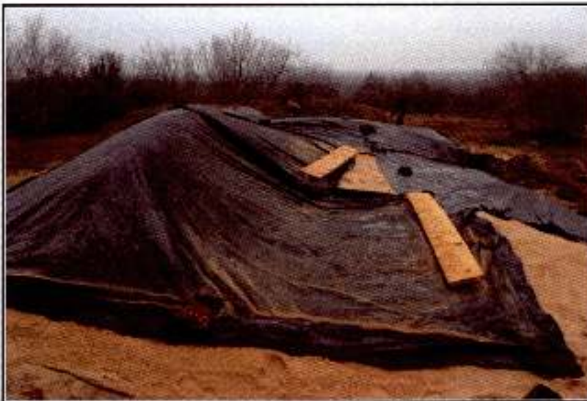
Figure 31. The north wall of Room 1 covered with geo-textile after the completion of the project, facing east.
