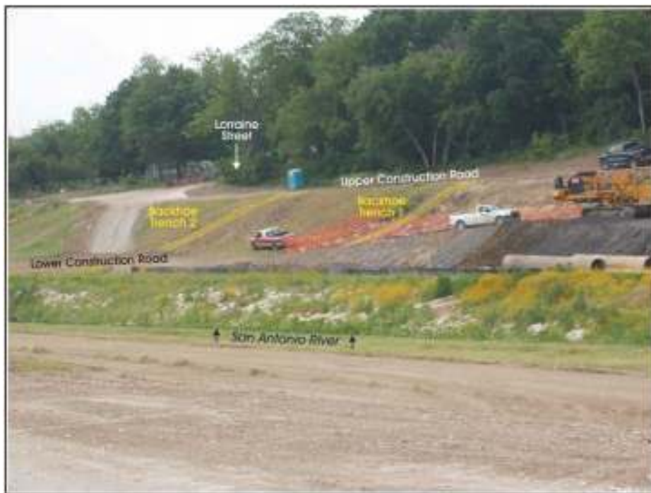
Figure 3-1. Area 1, seen from across the river, after Trenches 1 and 2 had been backfilled. Note the two levels of construction roads. The San Antonio River; not visible in this photograph, runs just below the line of concrete and limestone crossing the middle of the picture. Facing south-southeast.
