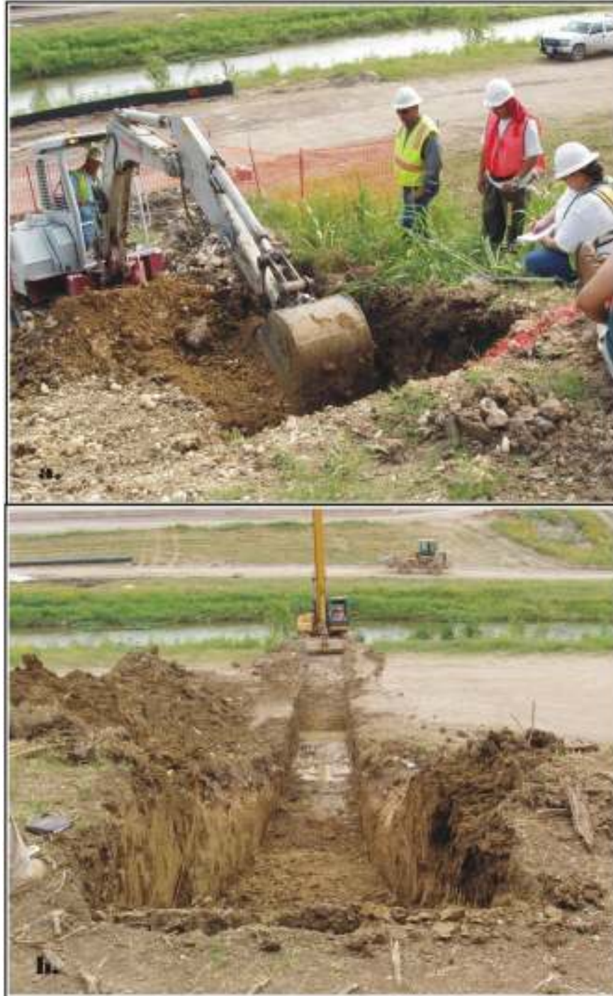
Figure 2-1. Digging trenches: a) Trench 1, near possible remnant of San José Dam, facing east; b) Trench 2, showing slope of trench bottom, water running into lower part of the trench. Facing northeast.
