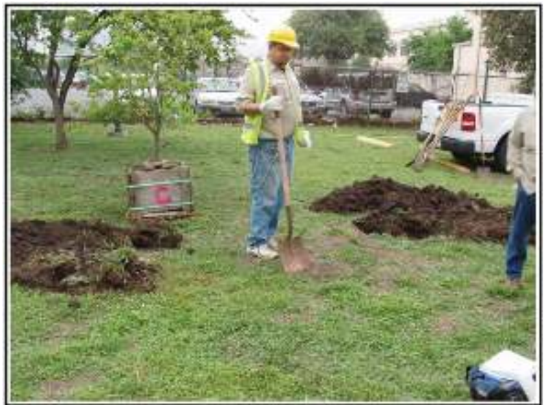
Figure 3-2. Moving Hole #2 after encountering an irrigation line. The final location is on the right. Facing North.
