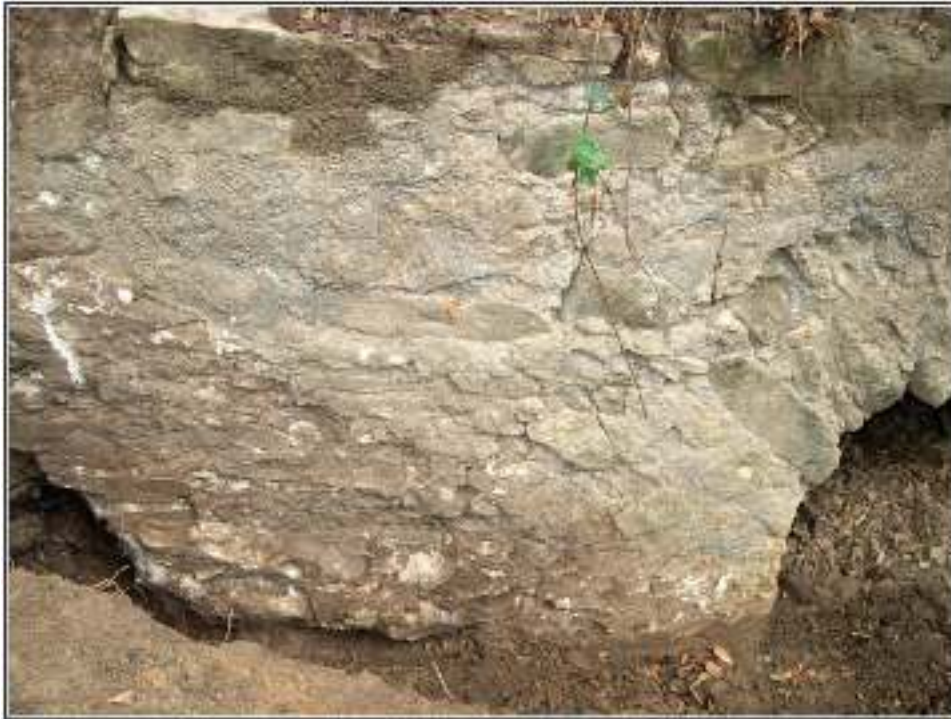
Figure 13. Base of the retaining wall along the north face of the arch.
