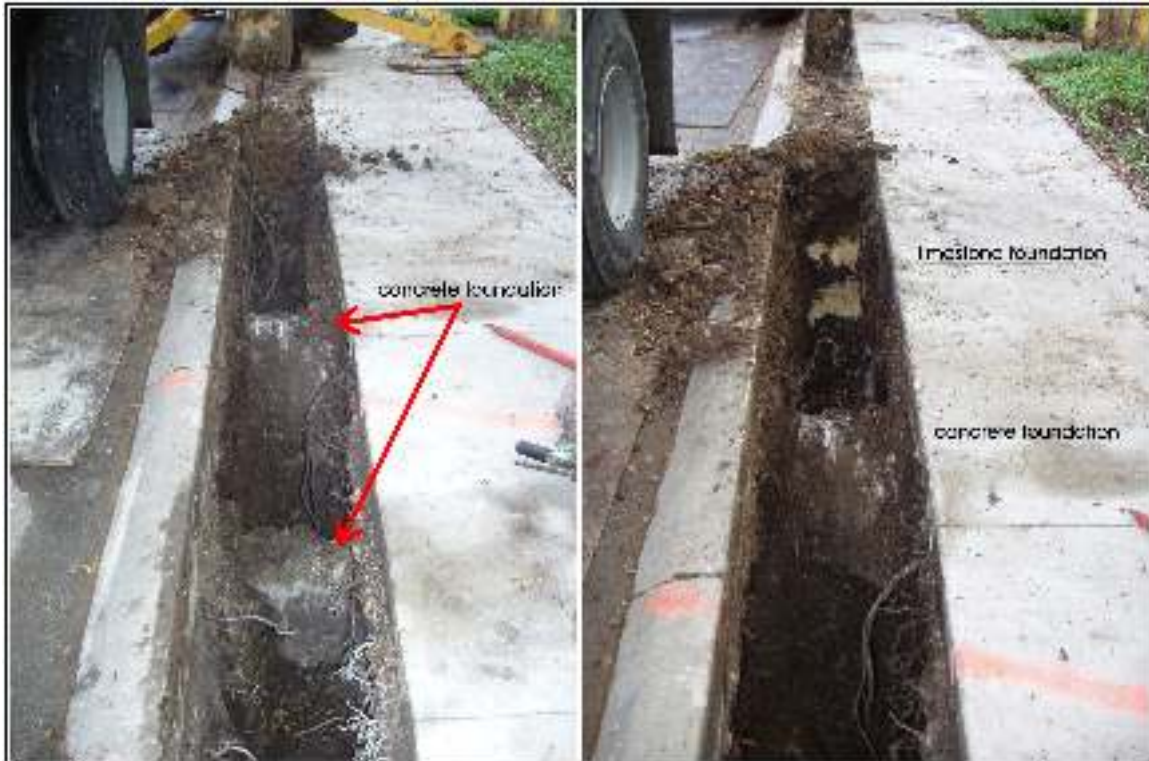
Figure 4-2. Excavation trench showing concrete foundation of shop building built in the early 20th century (left). Photograph (right) of limestone foundation of armory building built 1861 relative to that concrete foundation.
