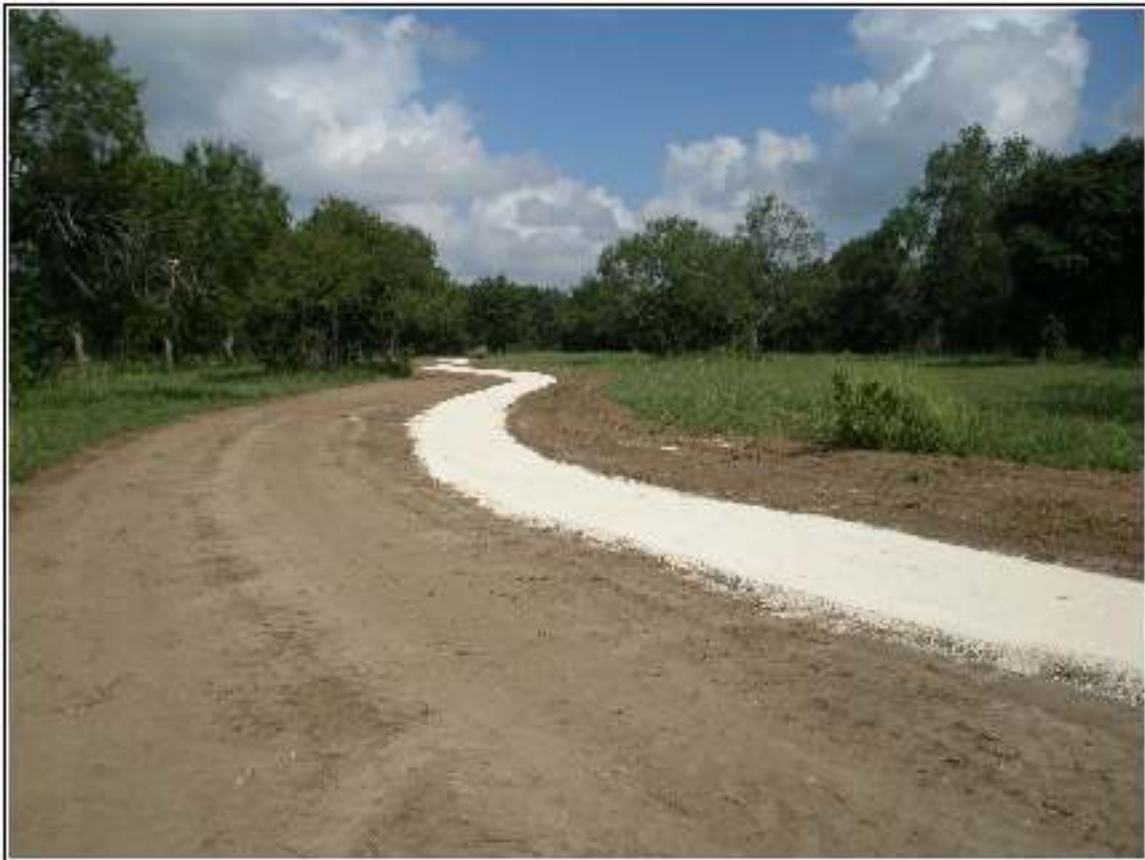
Figure 2-2. Trail easement that was graded prior to archaeological investigations northeast of the old development.
