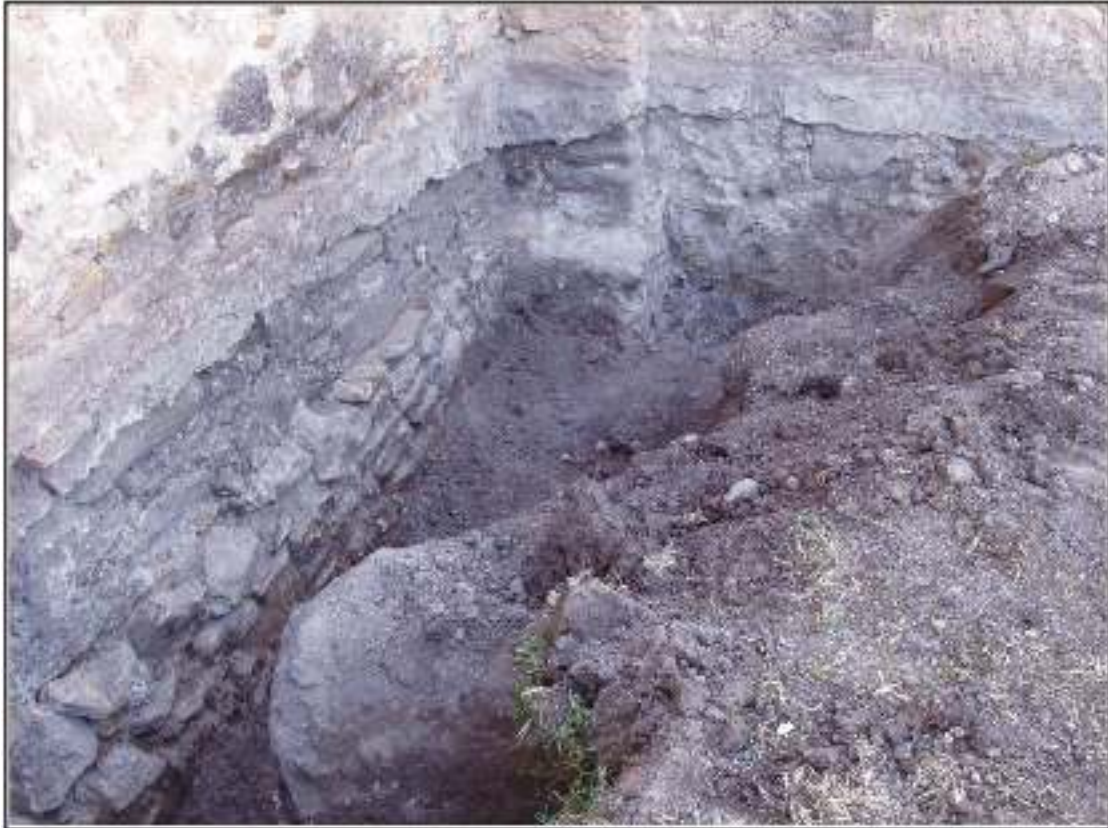
Figure 4-1. Photograph of soil removed from exterior of Church wall, west of the Rose Window. Facing northeast.
