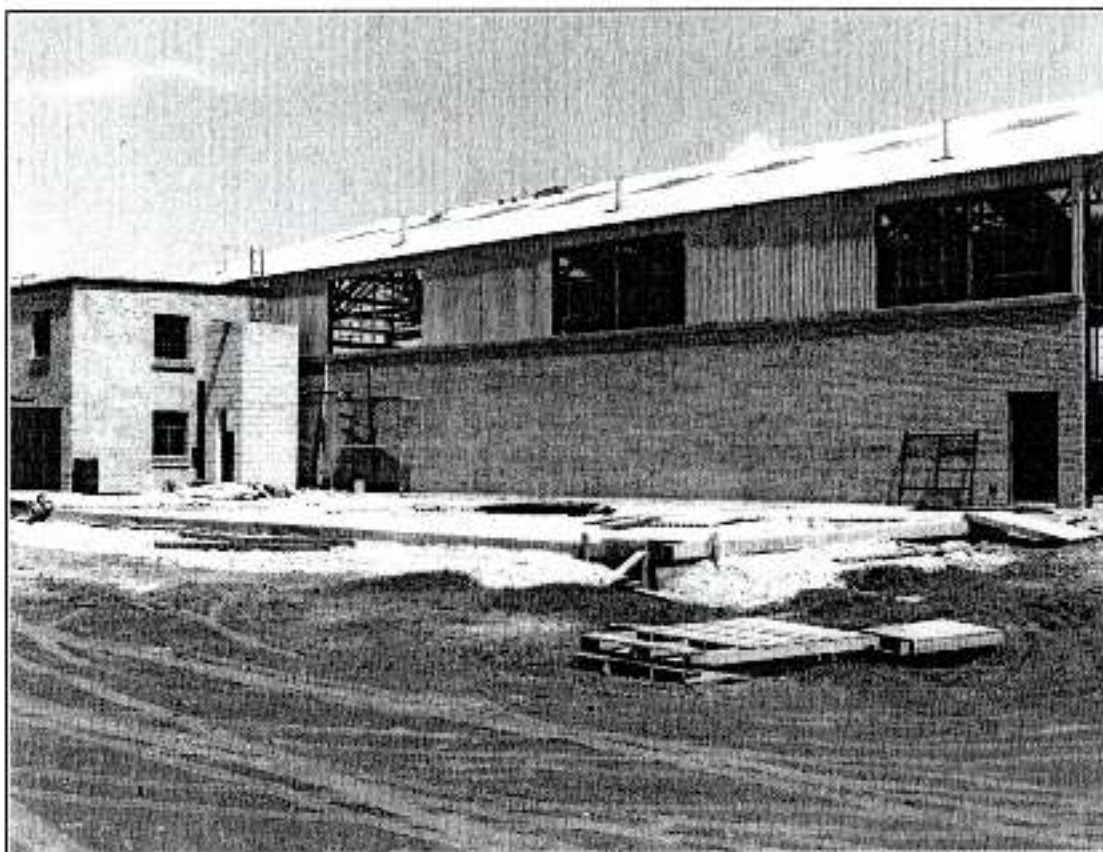
Figure A6. Construction of Hangar, photographed by Sgt J. T. Elsis, ANG Photo Lab, Kelly AFB, Texas Site of explosion, left.
