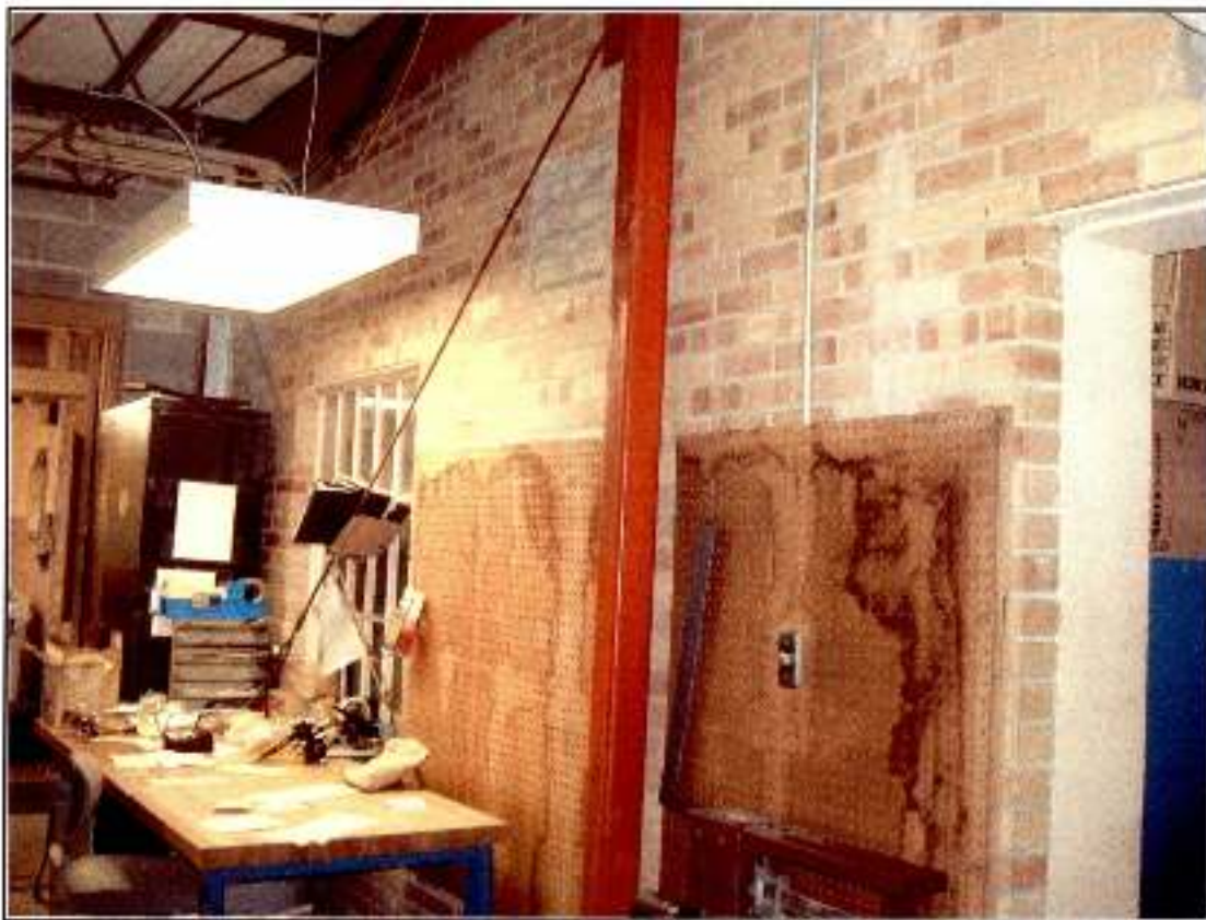
Figure 4-12. Exterior wall (now interior) rebuilt after the 1961 explosion, note exterior window still in place.
