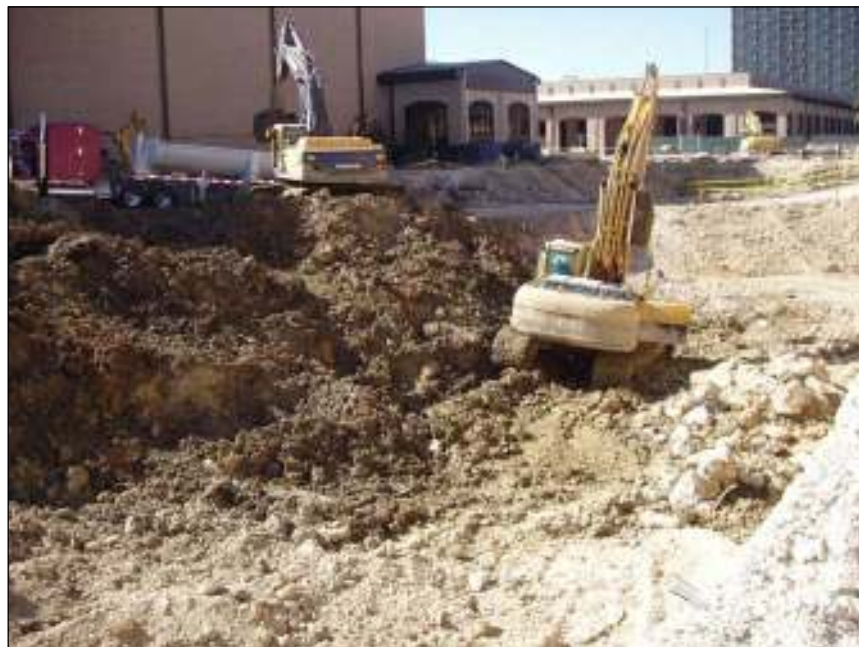
Figure 3-3. Photograph of mechanical excavation of the interior of hotel footprint, facing southwest.
