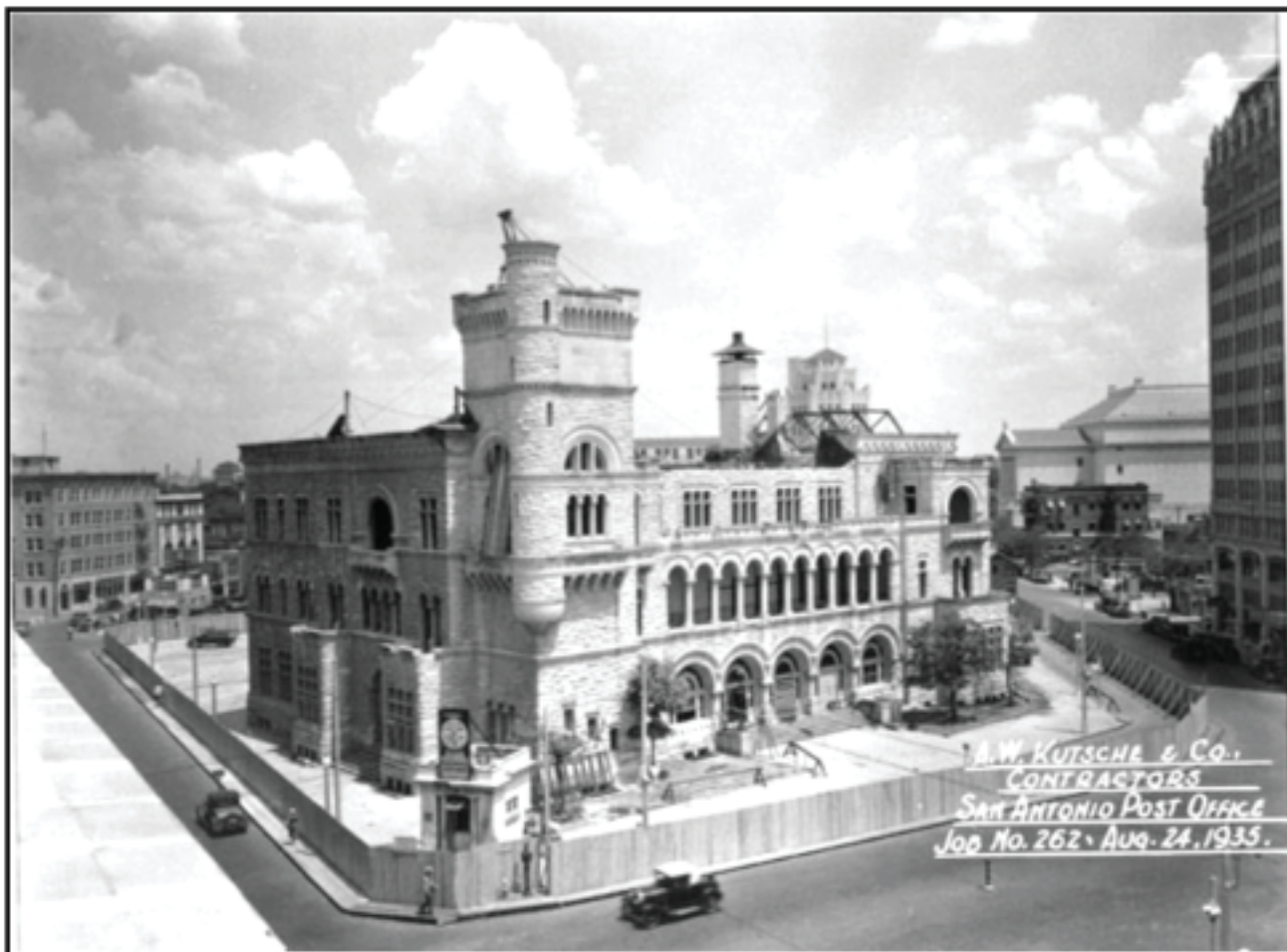
Figure 6-10. Demolition of the Federal Building and Post Office, San Antonio, Texas, August 24, 1935, University of Texas at San Antonio Special Collections Department, Digital Collections, General Photograph Collection, Image Number 101-0142. REDACTED IMAGE
