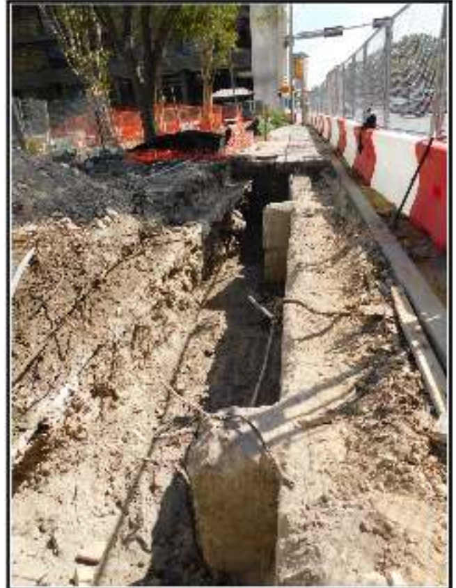
Figure 4-2. Electrical line project area along the east side of N. Flores Street. Note concrete pier and beam footings for the Majestic theatre, site 41BX2347 (view south).
