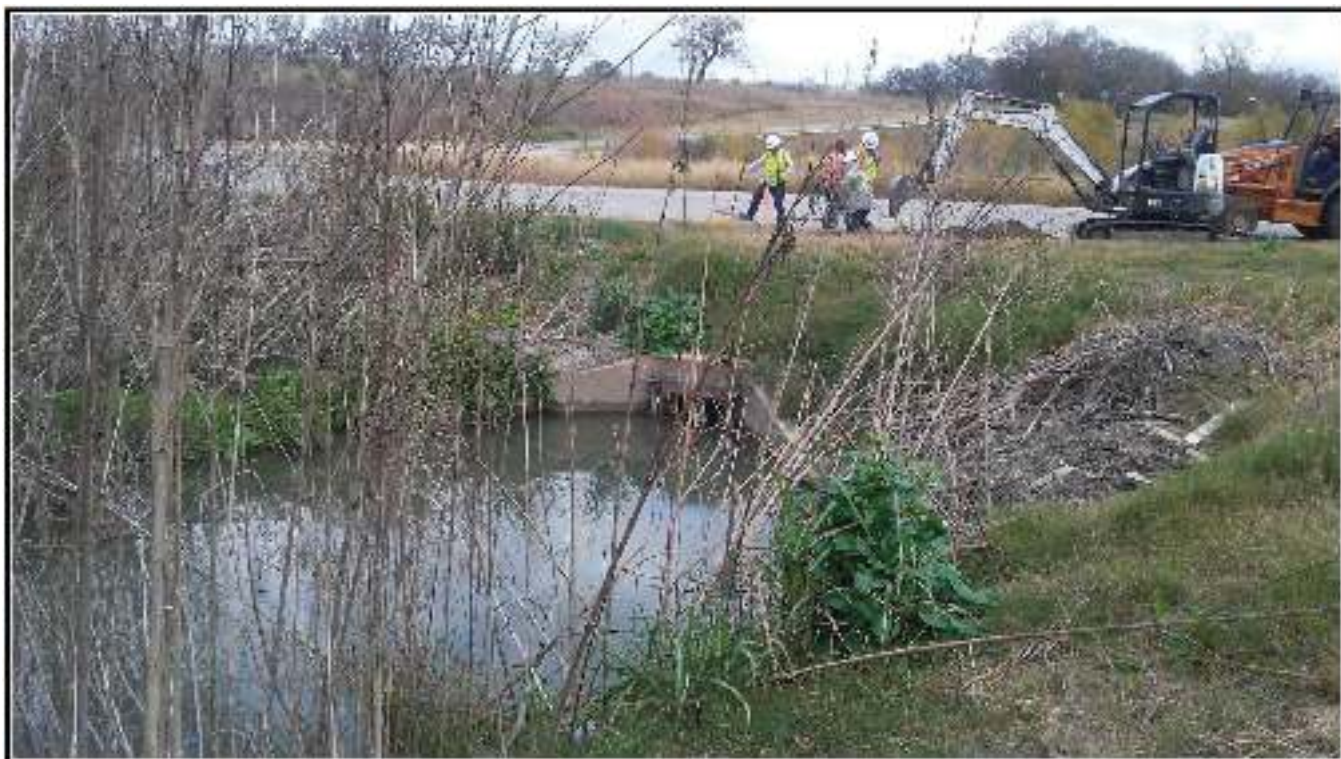
Figure 4-10. Acequia lateral culvert that runs under Camino Coahuilteca to the San Antonio River.
