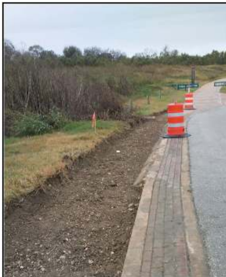
Figure 4-9. Excavations on Camino Coahuilteca for sidewalk installment, with existing sidewalks to the north.
