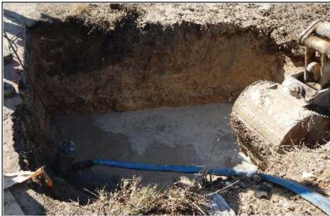
Figure 4-7. Flooded footing trench for pedestrian bridge crossing the San Juan Acequia. The layered appearance in the lighter portion of the soil profile is an artifact of the trench being repeatedly flooded and pumped during excavation. The profile did not exhibit this layering during the initial excavation.
