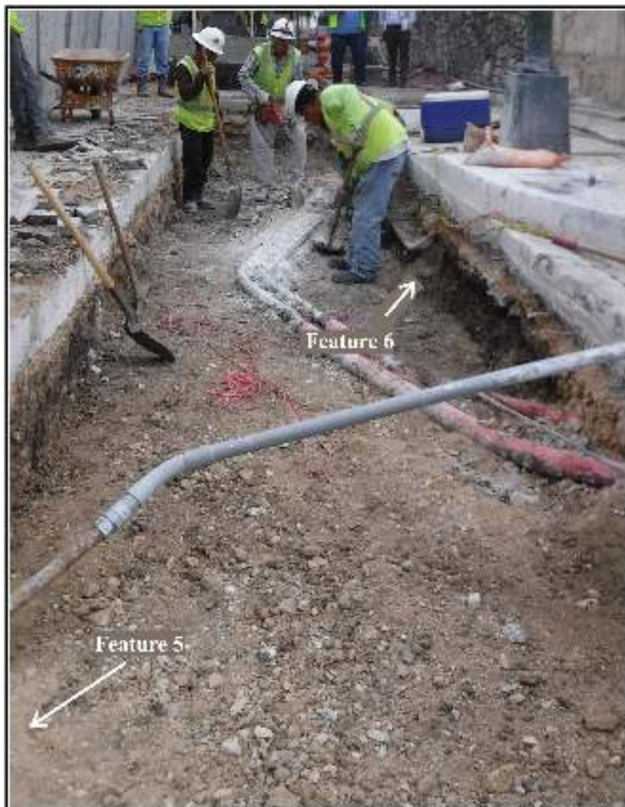
Figure 6-23. Area 6 demolition work in progress; approximate location of Features 5 and 6 (view east).
