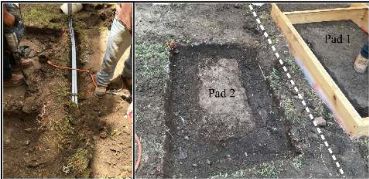
Figure 4-9. Left: excavation of Pad 1 with utility in place; view to the south. Right: completed pad excavation with dash line showing buried utility line.
