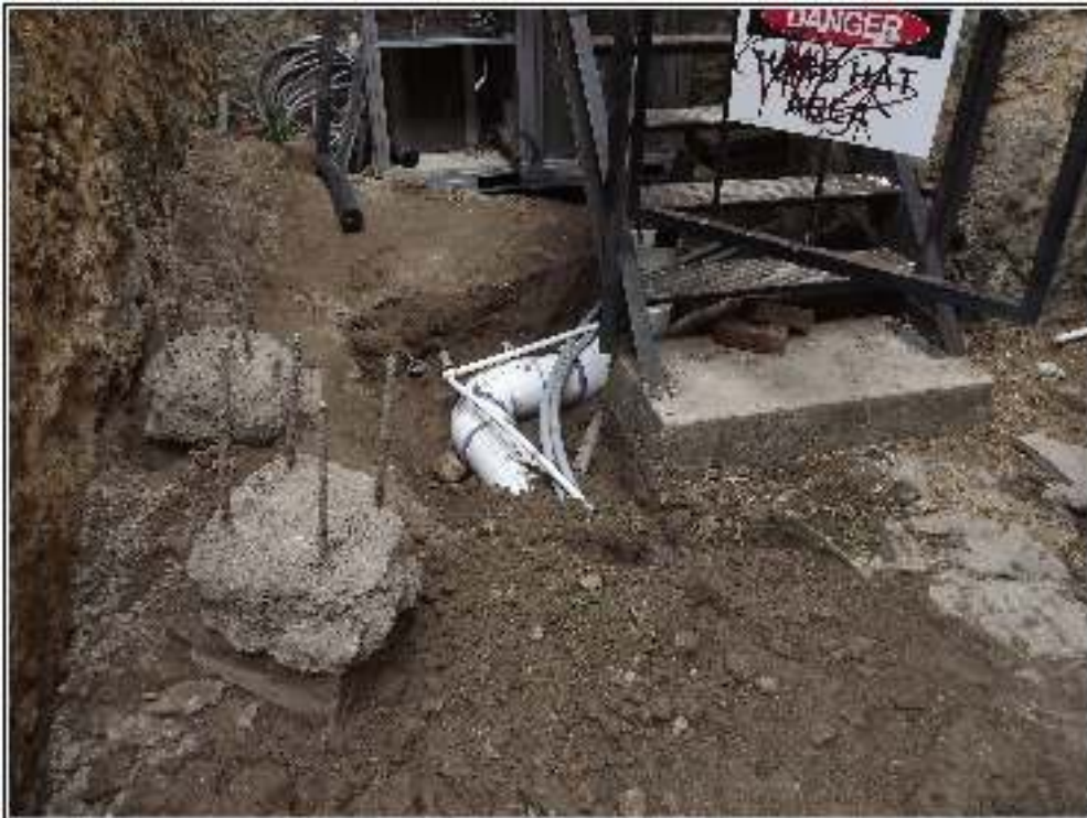
Figure 4-3. The completed excavation showing the new utilites running to the east under the stairs into the building. Concrete footings for the original air conditioning and heating units are on the left.
