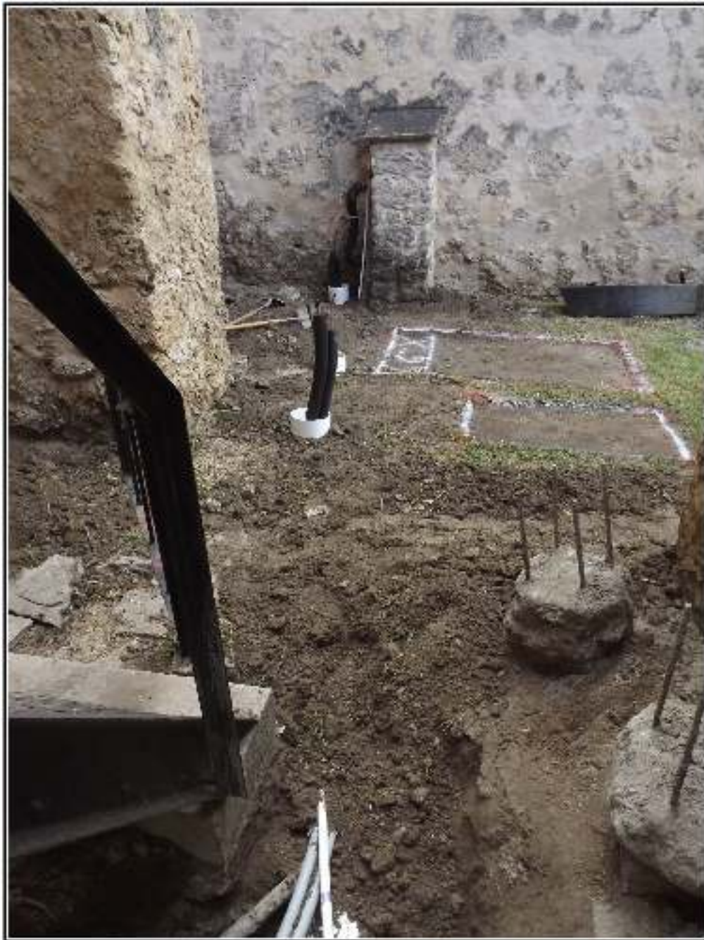
Figure 4-4. The completed excavation showing the new buried utilities running west into the church transept.
