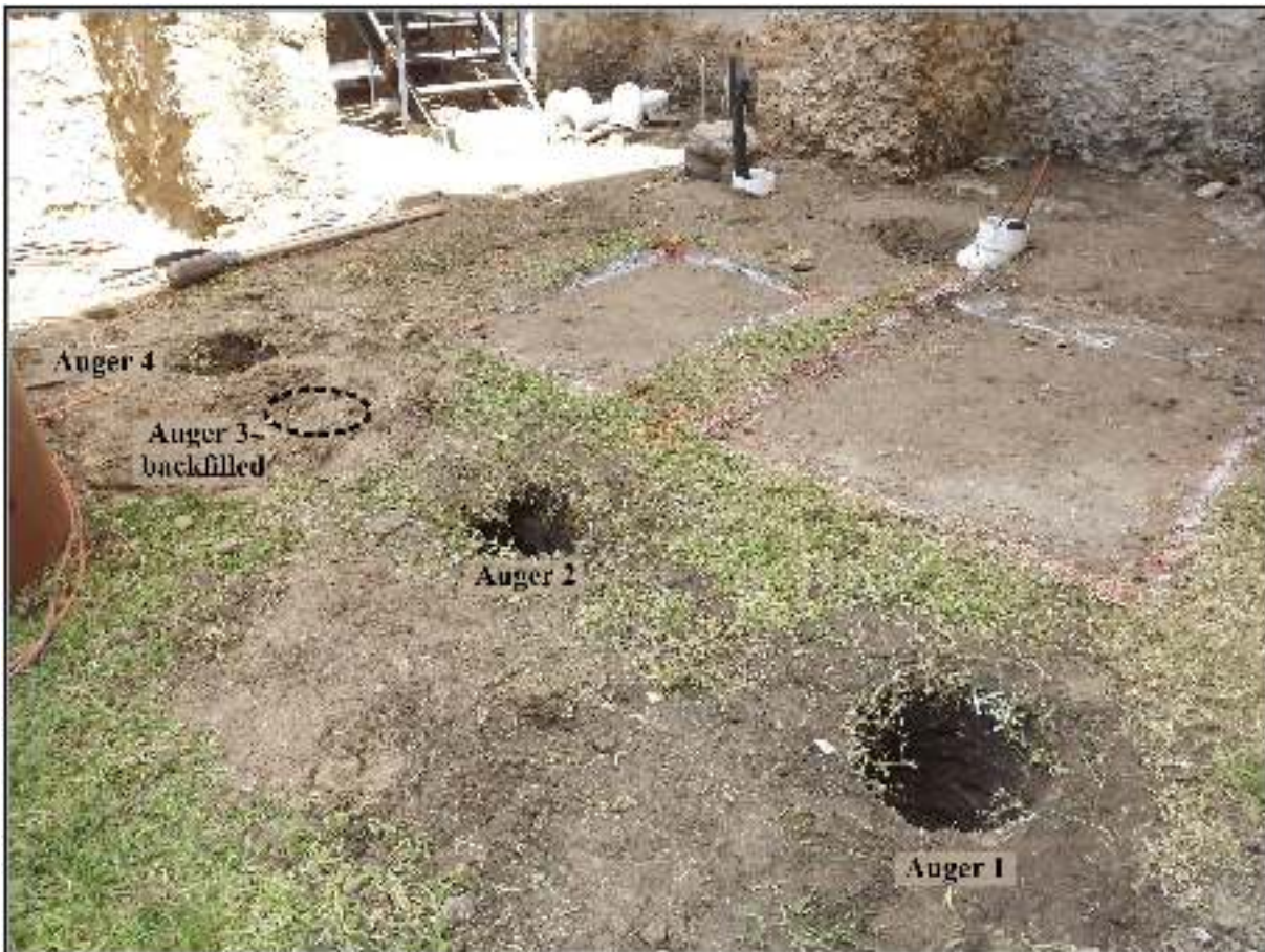
Figure 4-6. Location of auger excavations relative to church building and previous utility construction (view to the northeast).
