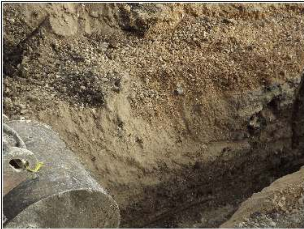
Figure 5-8. Utility trench profile, note a top zone of construction fill over clay.
