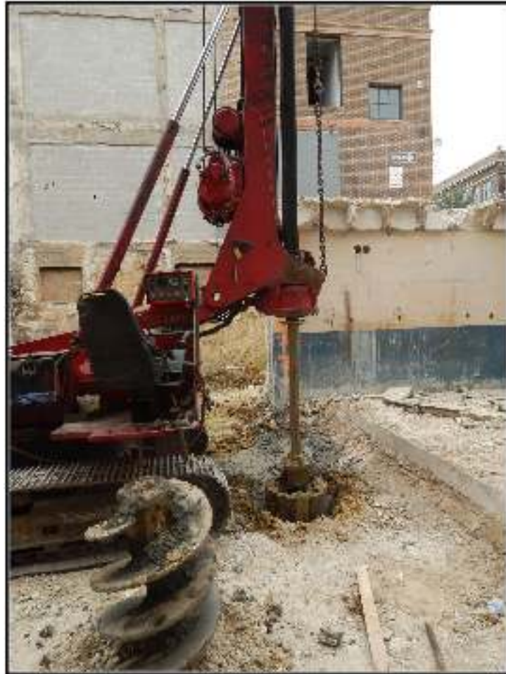
Figure 5-2. Location of pier hole starting surface; note that it is below the original ground surface.
