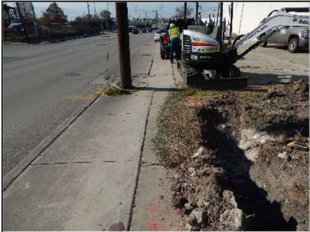
Figure 4-3. Gas line marking west of BHT 1 (facing west); north-south alignment marked in yellow spray paint.
