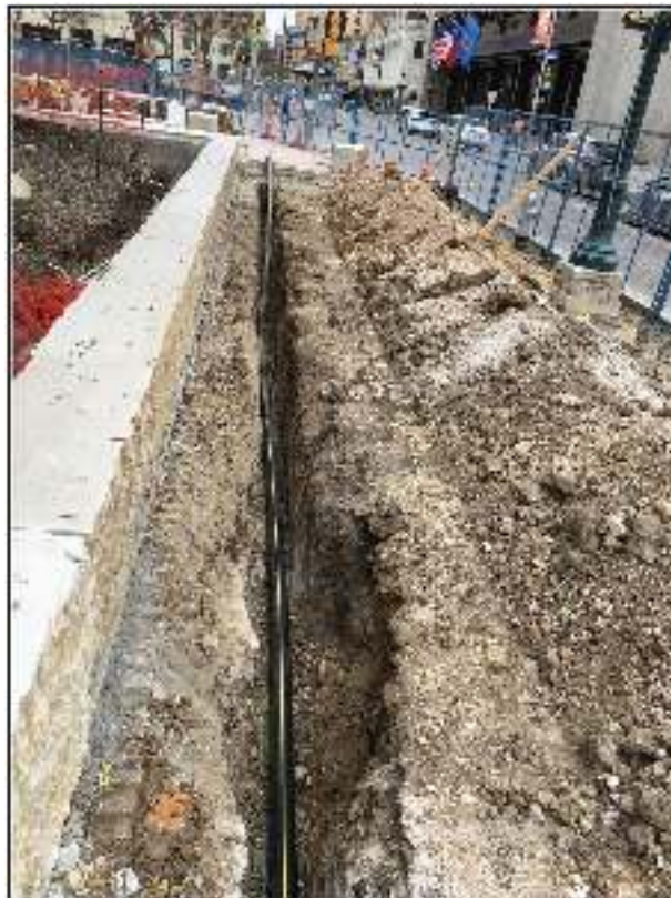
Figure 4-3. The eastern end of the CPS gas line trench with line installed.
