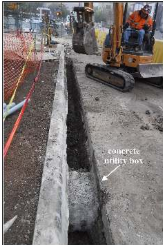
Figure 4-5. CPS electrical line excavations along the western end of W. Travis Street. Note the concrete utility box at the bottom of the picture indicating disturbances in this portion of the trench (facing west).
