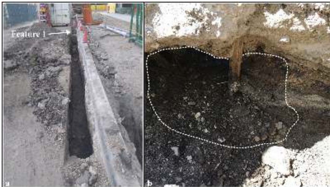
Figure 4-6. Feature 1, trash pit: a) location of the feature along Camaron Street and b) profile of the feature (facing east).
