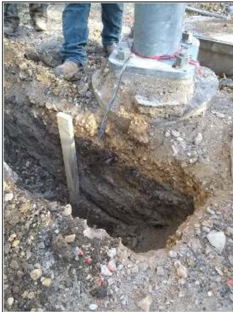
Figure 4-4. Trench excavation for the CPS electrical lines at corner of W. Travis Street and N. Flores Street. Note light pole and associated electrical box at upper right indicating disturbances in this portion of the trench (facing northwest).
