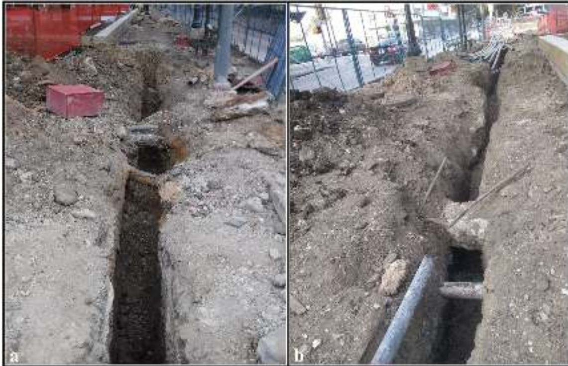
Figure 4-2. Excavation for the CPS gas line encountered: a) existing utility lines (facing east) and b) existing utility lines and concrete easements (facing west).
