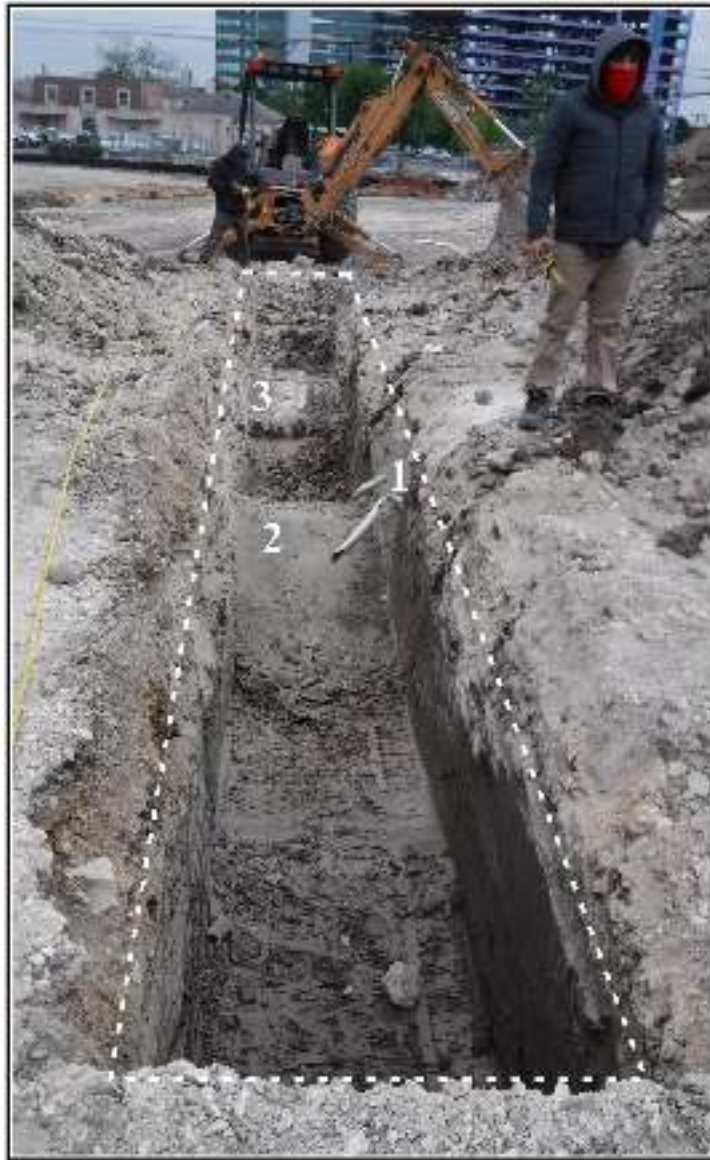
Figure 4-4. Backhoe Trench 1, excavation complete (view east): 1) irrigation lines, PVC; 2) concrete berm, possible duct bank; and 3) concrete pad.
