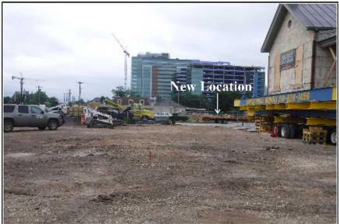
Figure 4-9. View of the house after being turned 180 degrees in preparation for move across the street (view east).
