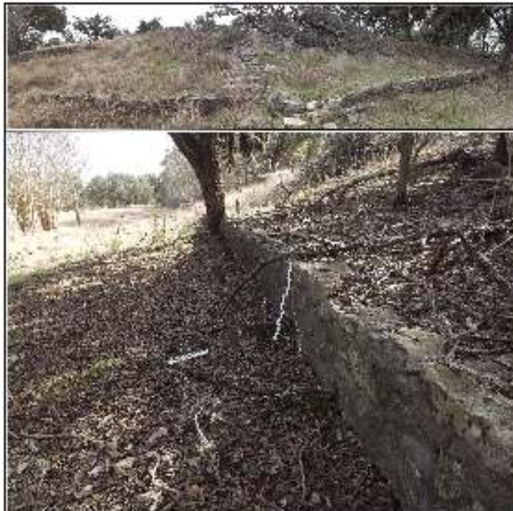
Figure 6-17. A view to the south of Feature 1 centered on the stairs (top). A view to the east of the lower segment of the terrace wall.
