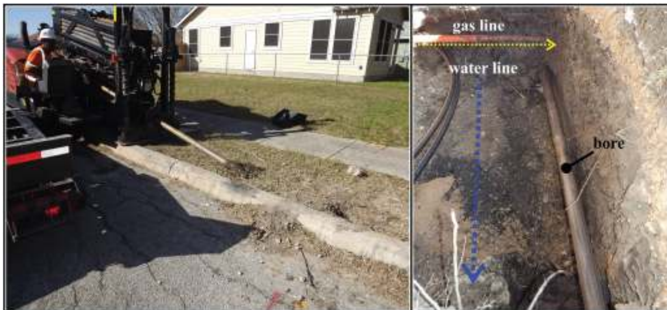
Figure 7-2. Image on the left shows the machine boring in to the test pit at Chihuahua and S. Colorado streets. The image on the right shows disturbance from past utility construction. The bore is below an existing gas line and to the right of a trench for a water line. The fiber optic conduits are in the upper left.
