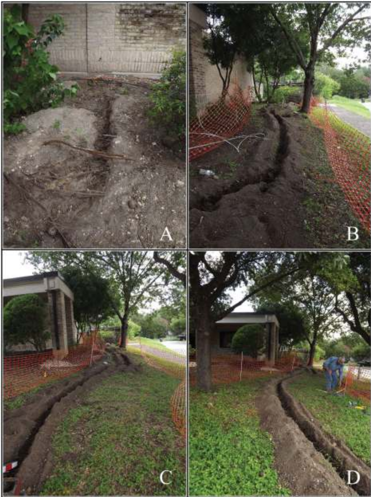
Figure 4-2. Views to the east showing trench location relative to the visitor's center. Image A shows the trench coming from the visitor's center. Images B and C show the trench location south of the building. Image D shows the trench termination at the sidewalk.
