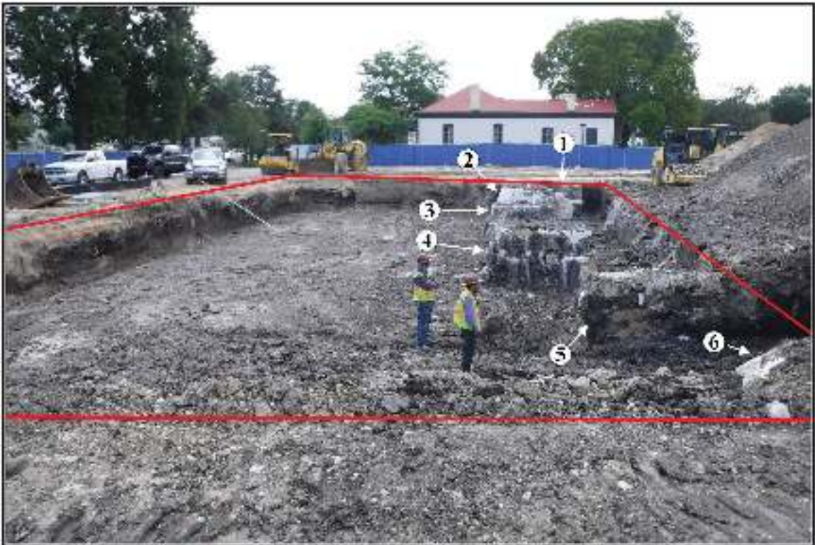
Figure 4-8. Excavated pit, outlined in red; note series of six concrete support piers. Koehler House (41BX592) in background, (view south).
