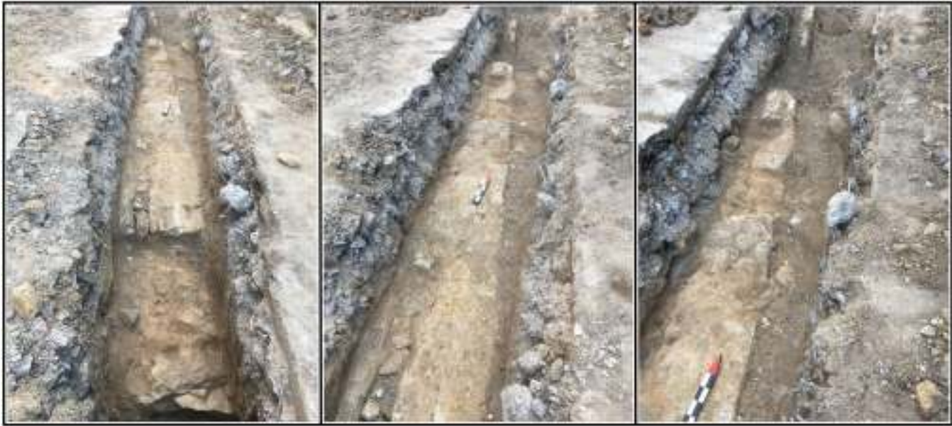
Figure 7-14. Feature 16 southern foundation walls of Bexar County Courthouse (41BX2165). Water line is to the east of the wall.
