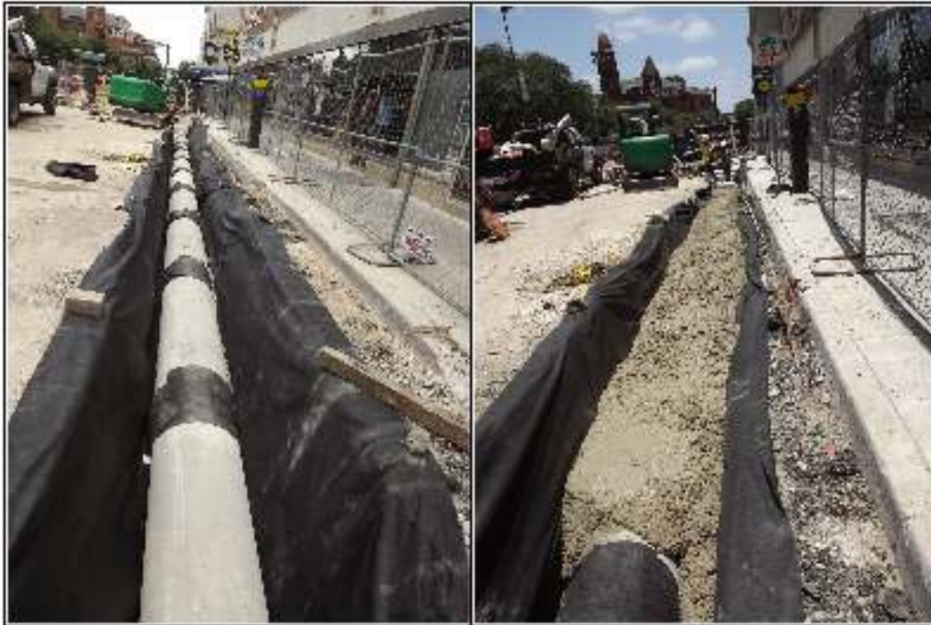
Figure 7-33. Image shows protection of acequia with geo-fabric to protect walls (left) and backfilled with flowable concrete (right).
