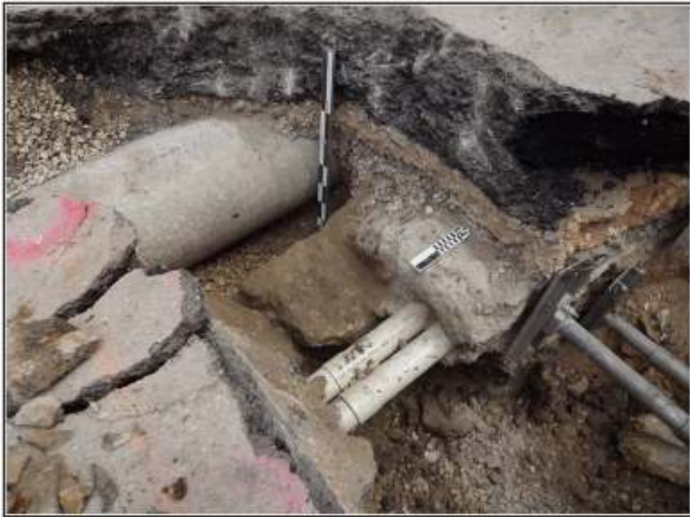
Figure 7-24. Photo of the east wall of the San Pedro Acequia just north of the intersection of N. Main Avenue and Commerce Street. The east wall has at least one course removed with a cable duct bank encased in concrete laying on top of it.
