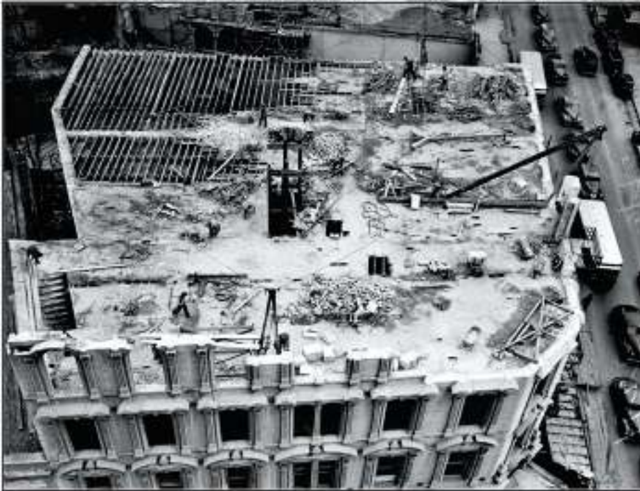
Figure 5-25. The demolition of the Kampmann Building (San Antonio Light Photograph Collection, UTSA Special Collections, L-2291-F).
