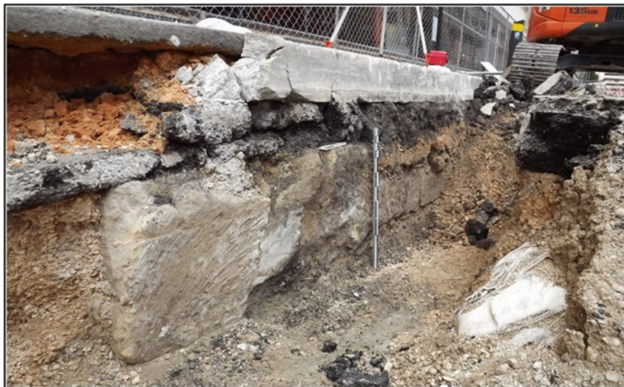
Figure 7-27. West wall of acequia showing depth to floor from street level (top of asphalt).
