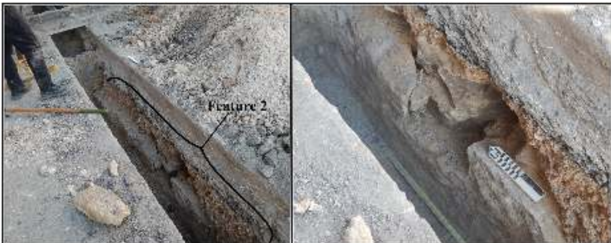
Figure 7-7. Feature 2 (left) found during excavation for a gas line at Commerce and Soledad streets; trench width approximately 60 cm (23.6 in.). Detail (right) of limestone wall.
