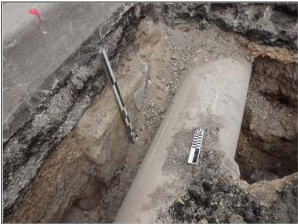
Figure 7-25. Photo of the west wall of the San Pedro Acequia at the same location as shown in Figure 7-18. The west wall is located mostly under the sidewalk on N. Main Avenue with the current storm line laying in its channel.
