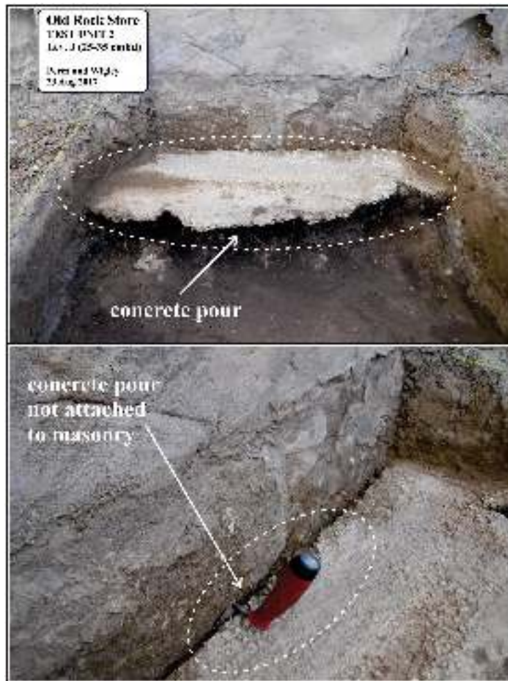
Figure 4-3. Close-up photos of TU 2; note concrete pour meant as a water barrier.
