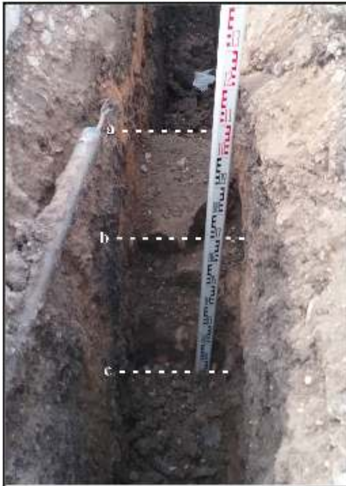
Figure 5-13. Feature 4, stone foundation, facing south. Horizontal extent of feature shown between lines a and b. Vertical extent of feature shown between lines b and c. Scale is metric.
